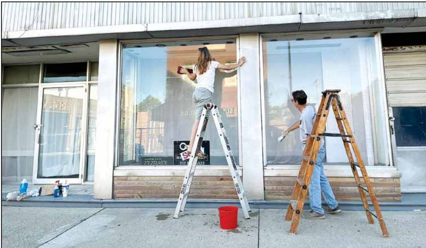
Above, Chris and Terri Casey clean the windows lining the Corner Block shortly after taking ownership of the building.
