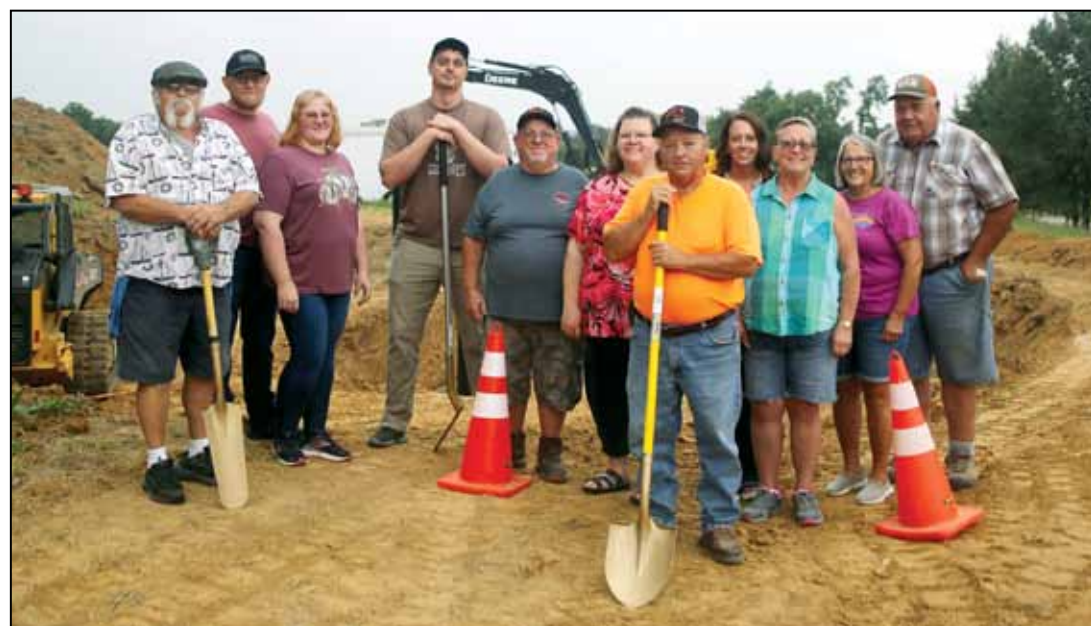
Breaking ground for the new Butler water tower, from the left are Trustee Cary "CB" Cunningham, Kyle Mathenia, Trustee Cathy Shepherd, Trustee Darrell Damm, Bob Lane, Village Clerk Kendra Lane, Mayor Rickey Lane, Trustee Rachel Cunningham, Trustee Debbie Beeler, land owners Jean and Tom Anderson. Not present: Trustee Rachelle Shepherd.
