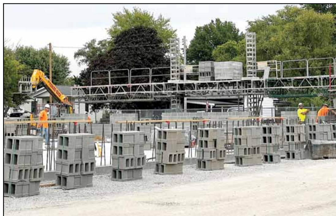
Construction crews work on the storm shelter as part of the new Litchfield Primary School construction project. Formerly JD Colt Elementary School, the new building will house pre-K through first grade students in the district. It's expected to be completed for the start of the 2024-2025 school year.
