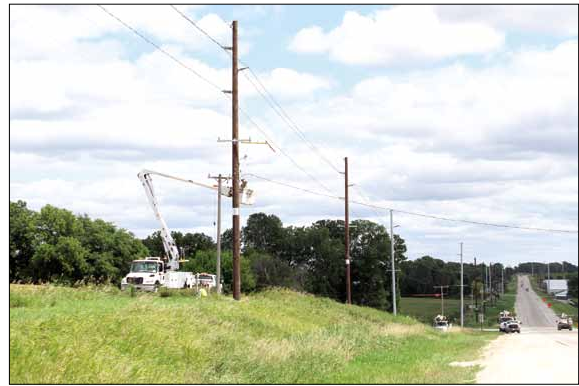
Crews from ITC Midwest string new power lines along Highway 22 between Kalona and Riverside. KALEN MCCAIN/THE NEWS
