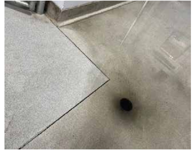
A recent photo of backed-up drain at the shelter.
