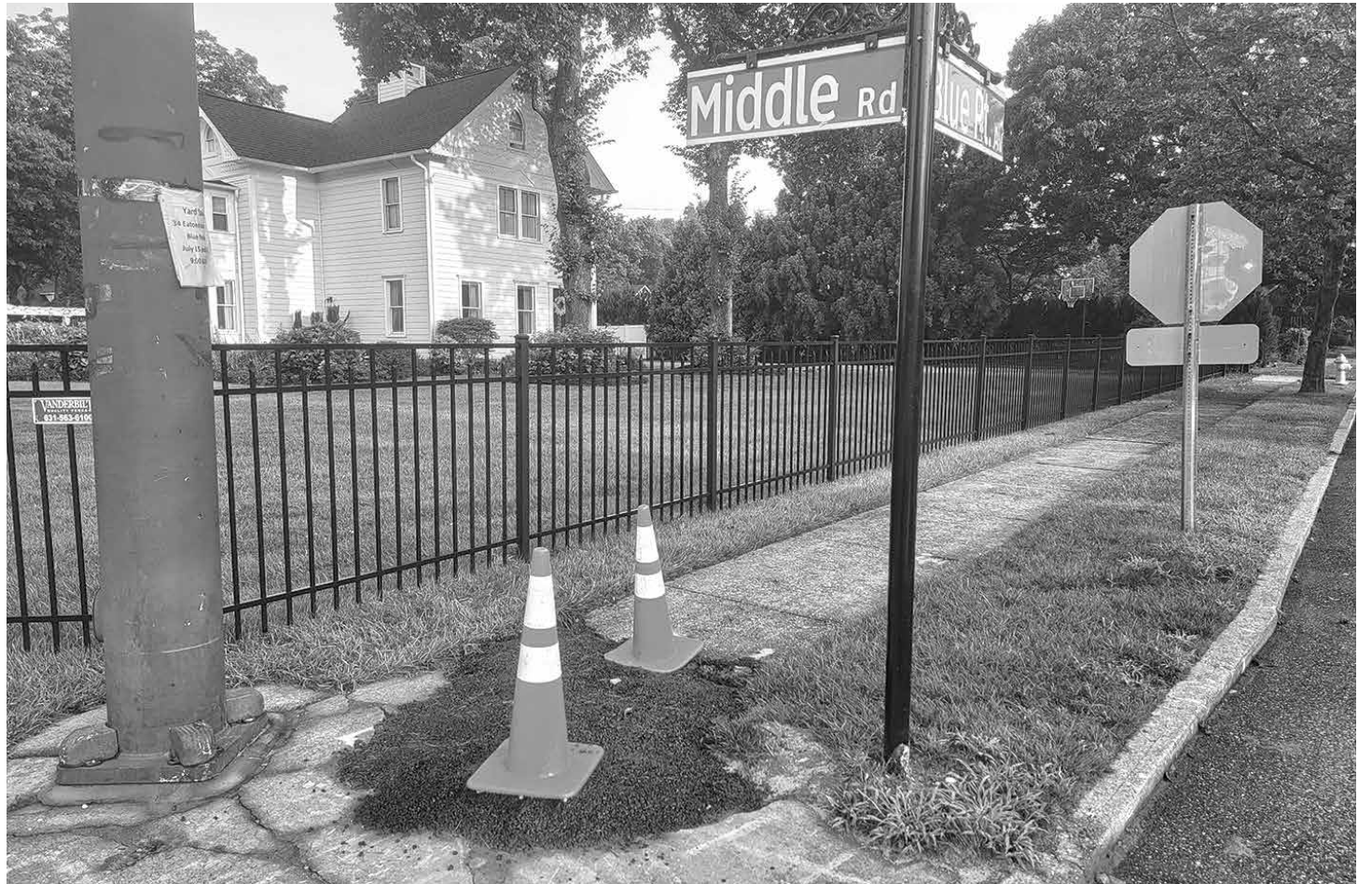
National Grid began replacing gas mains in spring after receiving a permit from the Town of Brookhaven and is slated to complete the project involving Blue Point Avenue and Danes Street by this fall. SCN/Desmond
