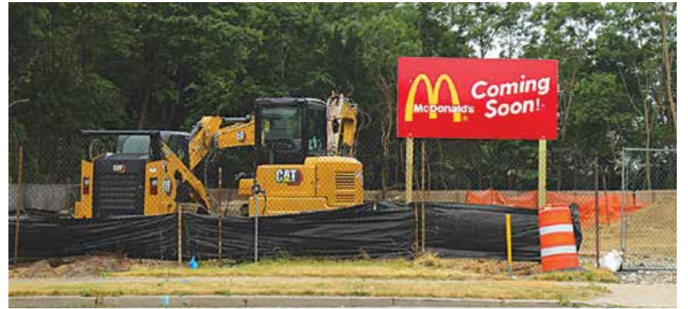
With demolition completed in under a month, new construction on the McDonald's on Montauk Highway in Blue Point is estimated to take four months to complete.
