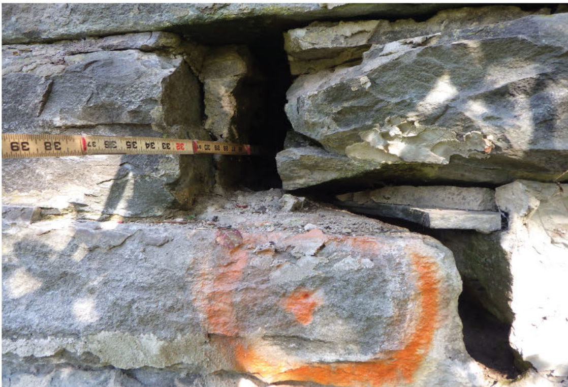
16. Deep void and loose stones at the Far Right Wingwall.
