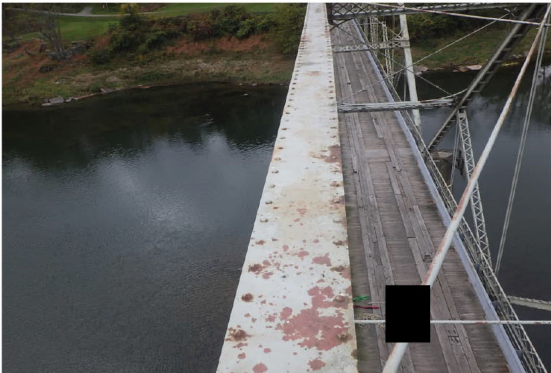
24. Typical top chord condition, U2-U4, Right Truss in Span 2.
