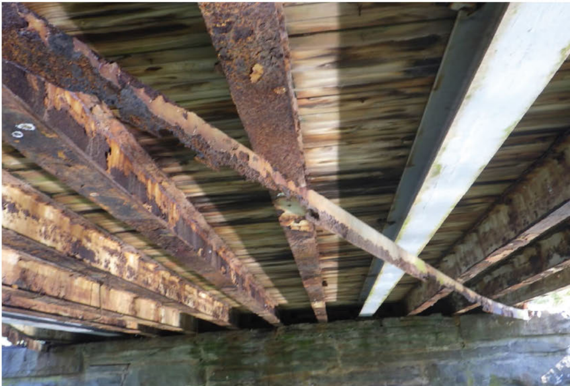
66. Sagging right lower lateral brace, Bay 12 in Span 1. (Removed during inspection)
