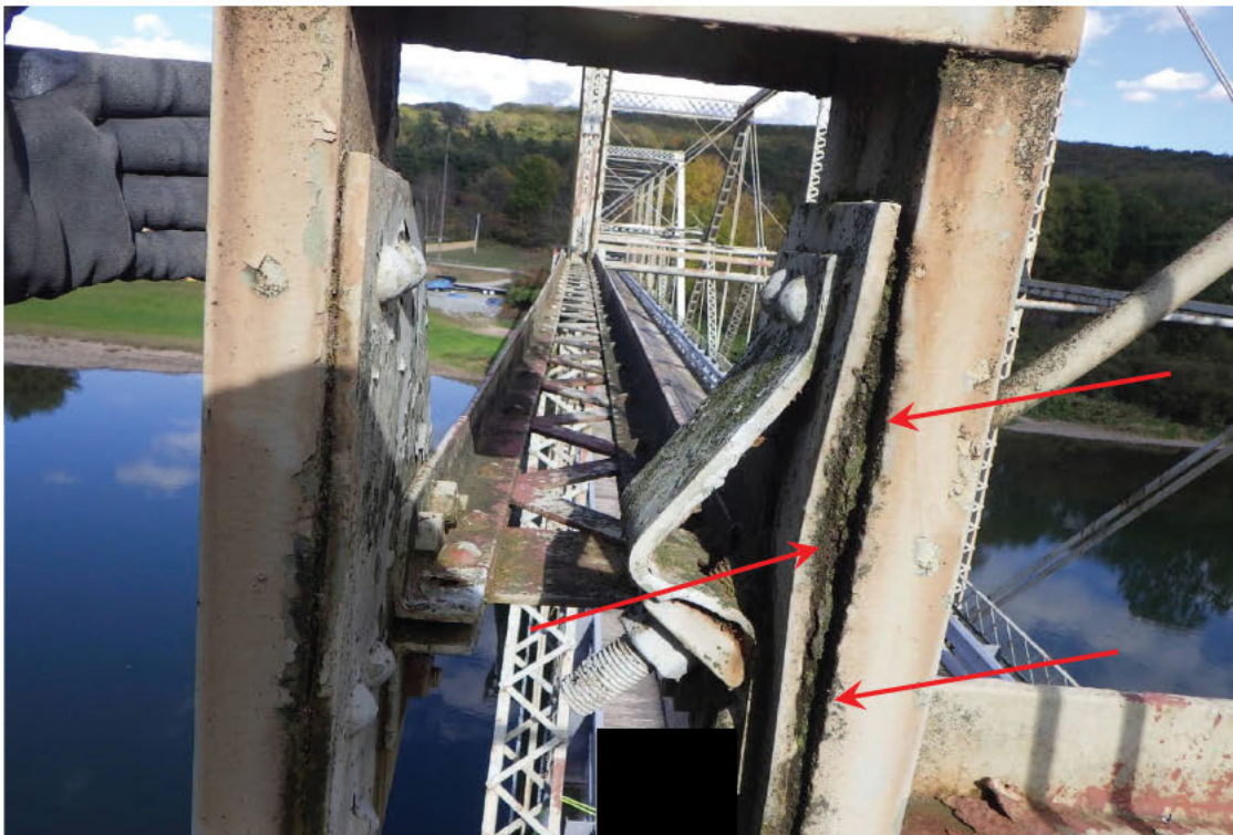
36. Pack rust between L4-U4 & M4-M5 at M4, Left Truss, Span 1.
