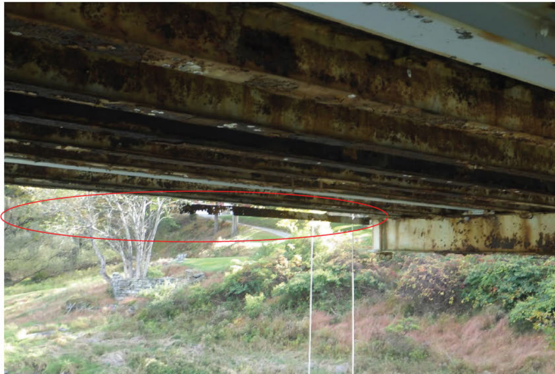
64. Partial length missing and cantilevered lower lateral bracing, Bay 6 in Span 1, looking right.
