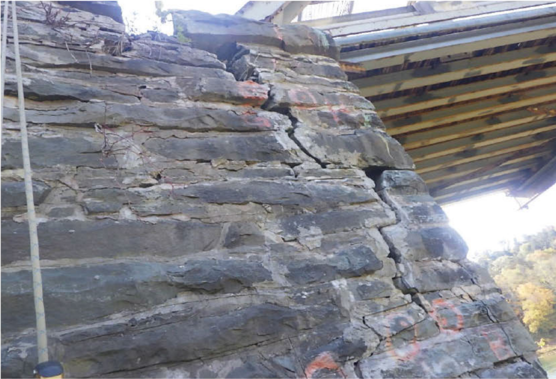
119. Deep void in crack with loose stones and fill at the Far Left wingwall.
