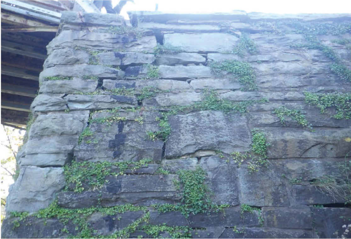
7. Near Left wingwall with loose and fractured stones with adjacent mortar joint voids
