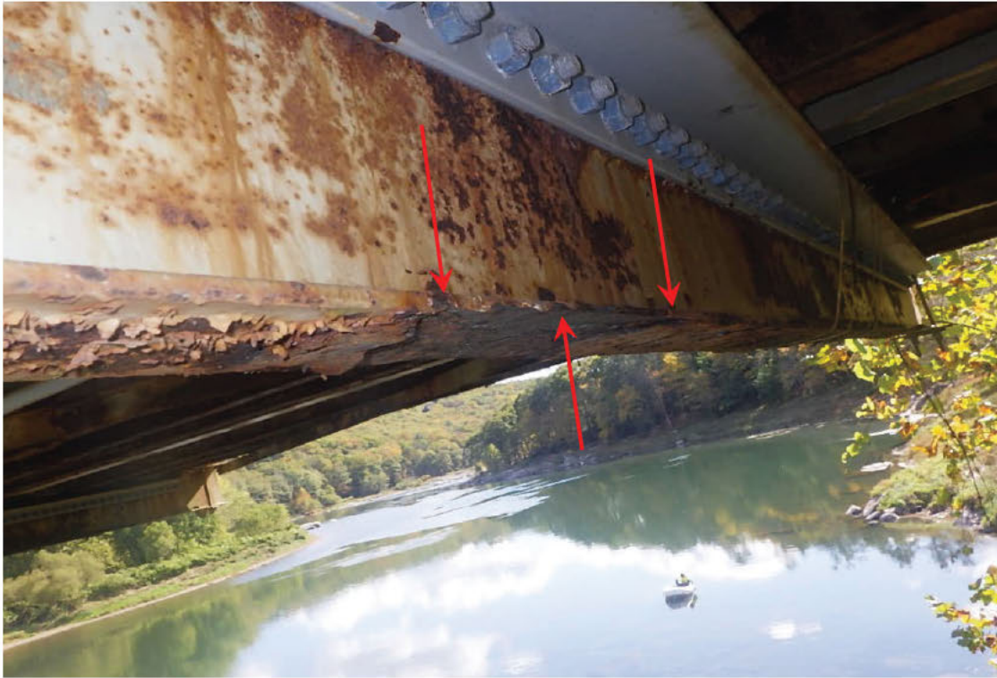
49. Section loss to bottom flange of Floorbeam 1, Span 1, looking right.
