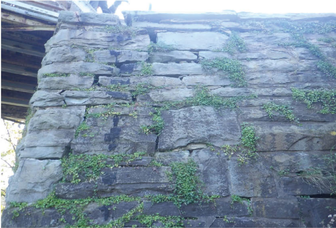
95. Fractured cap stone and deteriorated mortar at the Near Left wingwall.
