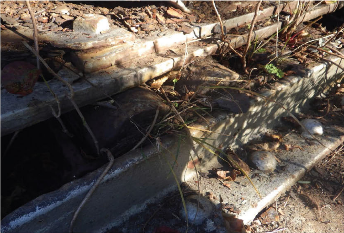
85. Exposed rollers with debris impacting movement of the Right bearing at the Far Abutment.
