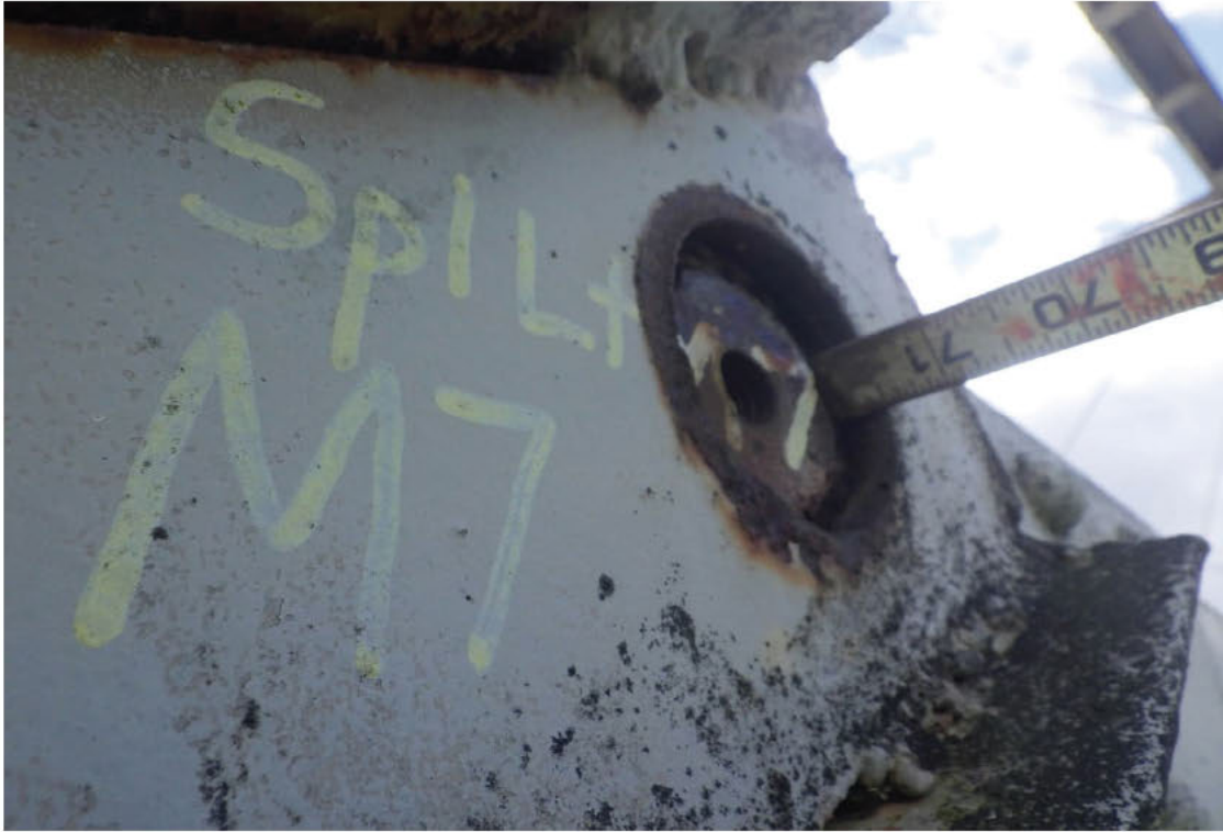
35. Pin plate not bearing on pin for M7-L8 at M7, Left Truss, Span 1.
