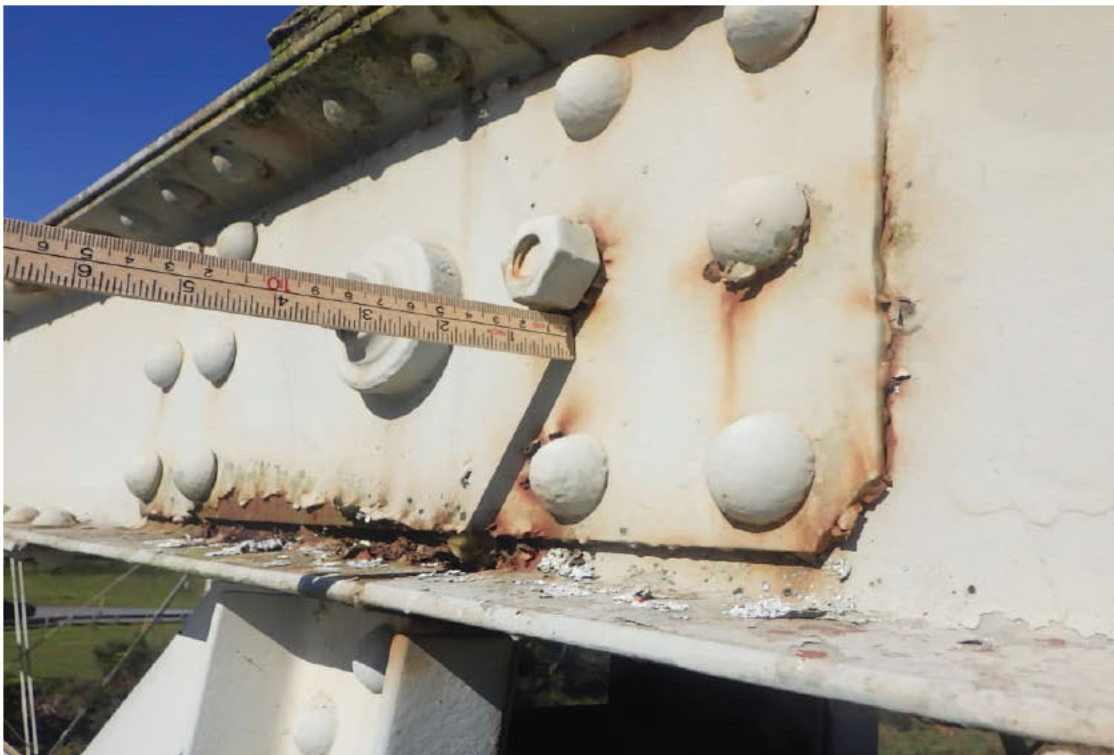
40. Un-seated bolt at U8, Right Truss, Span 1.
