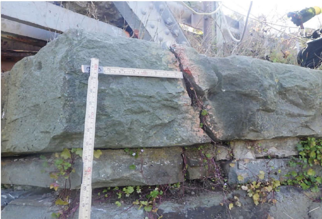
8. Fractured cap stone at NAB/NL Wingwall interface.
