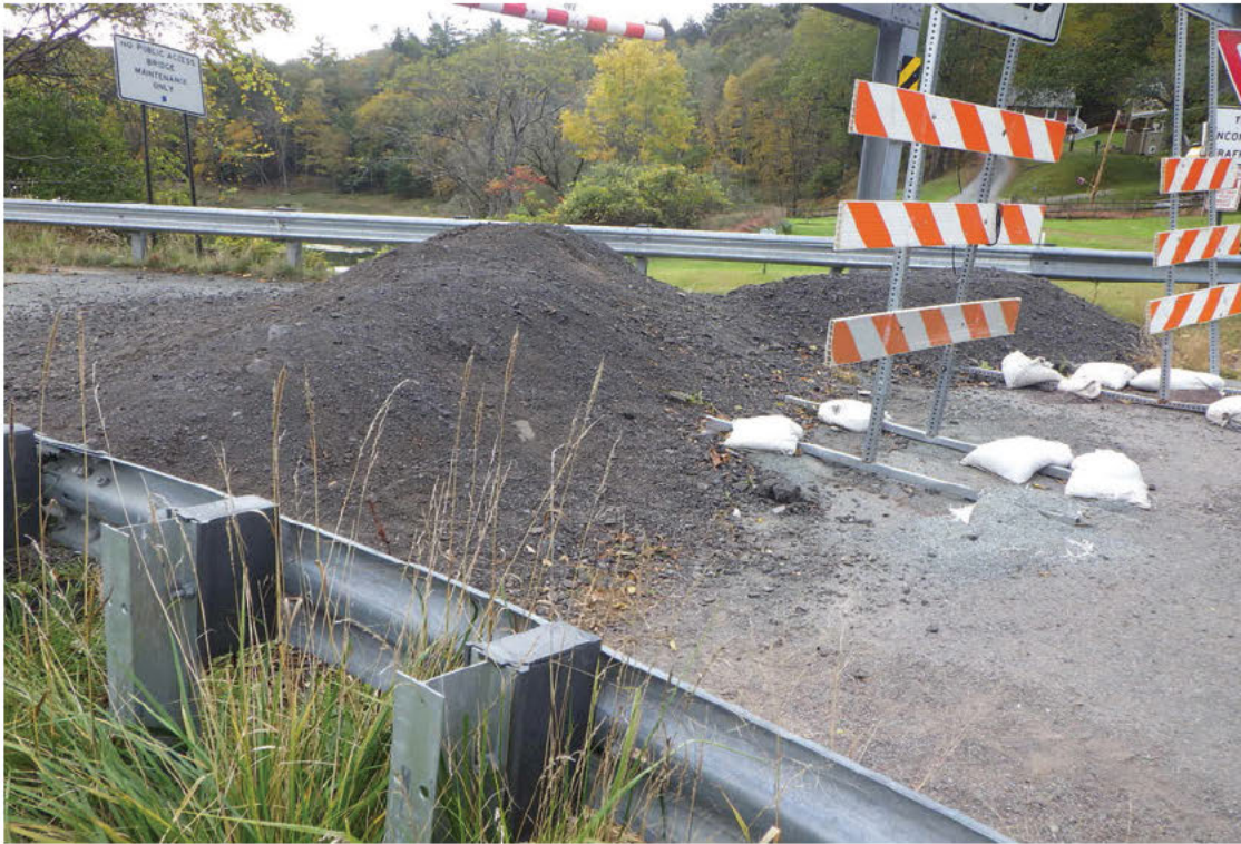
9. Typical gravel dumped at the ends of the bridge.
