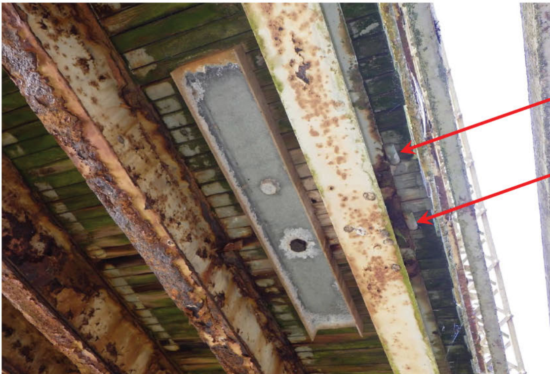
18. Typical bridge rail anchor not engaging stringer top flange.
