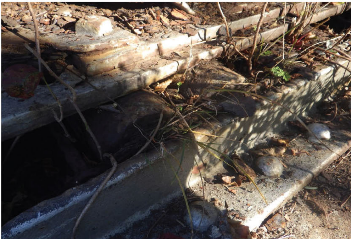
4. Close-up of previous photo showing exposed rollers.
