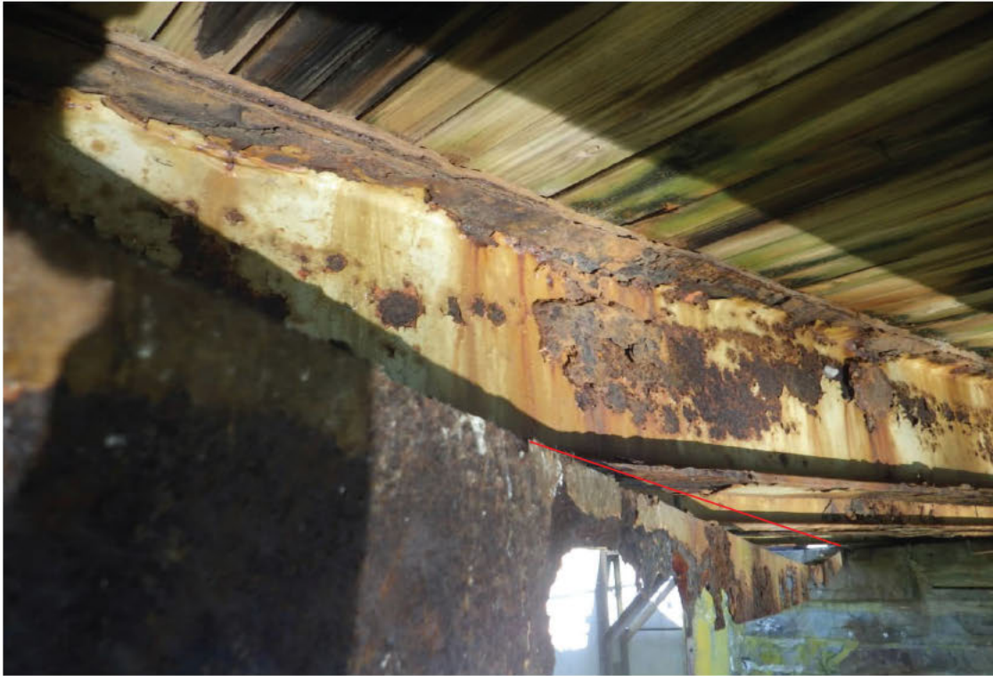
63. Sagging lower lateral bracing on left side, Bay 12 in Span 1.
