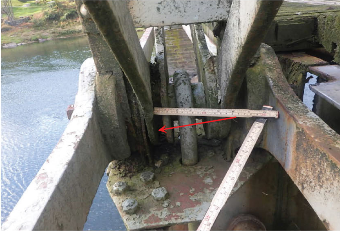
31. Diagonal eyebar with section loss, L6-M7, Right Truss.
