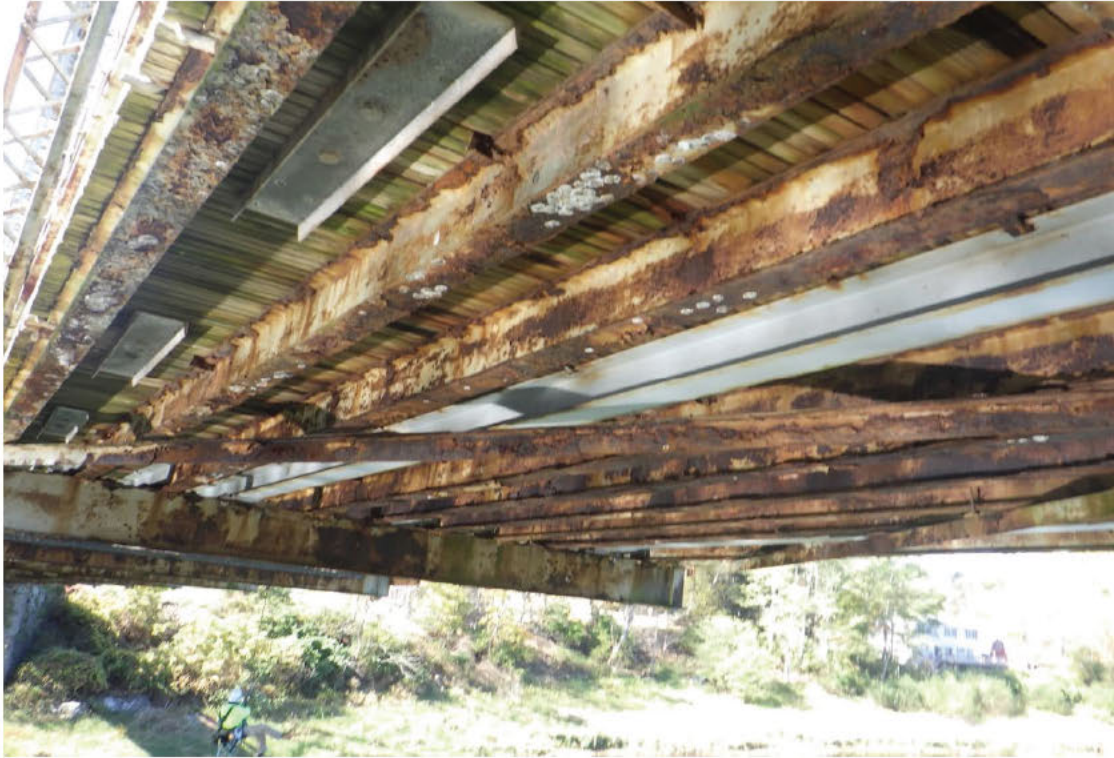
53. Typical stringer condition in Span 1 between Floorbeam 10 & 11, looking back.
