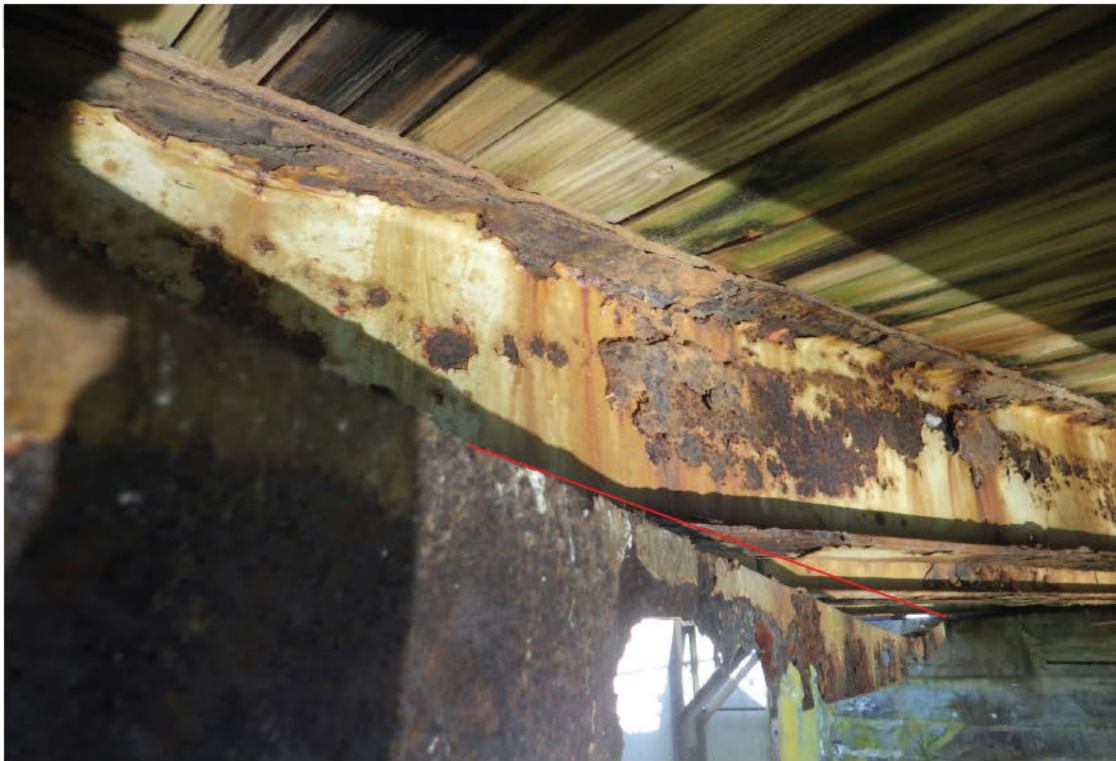
20. Deflected left lower lateral brace with severe corrosion, Span 1 between FB 11 & 12, looking ahead.
