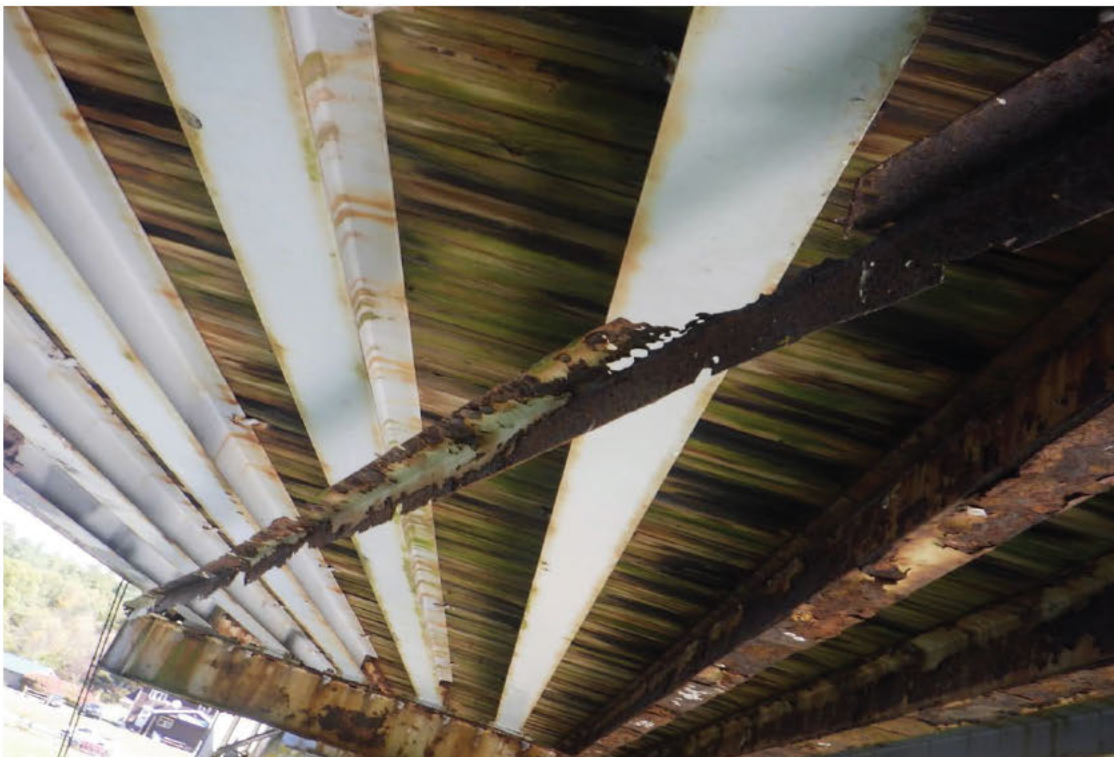
62. Severe section loss to left side lower lateral bracing, Bay 10 in Span 1.
