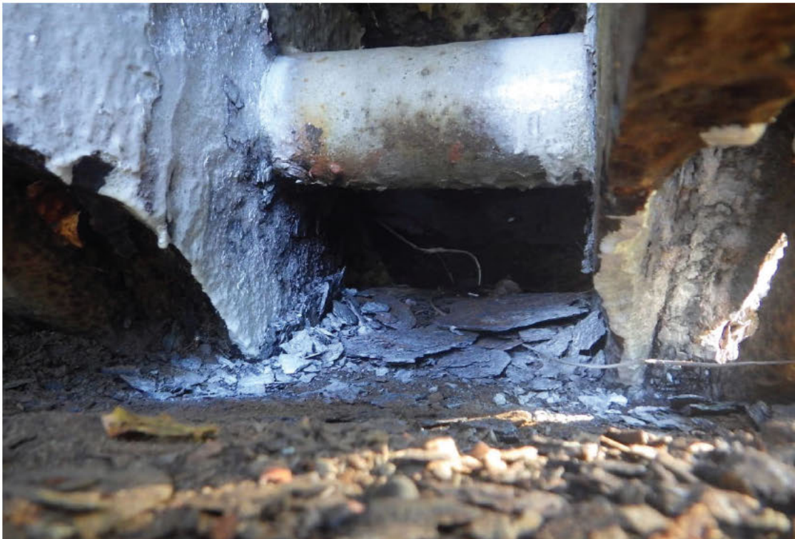
28. Close-up of previous photo showing section loss to eyebar head.
