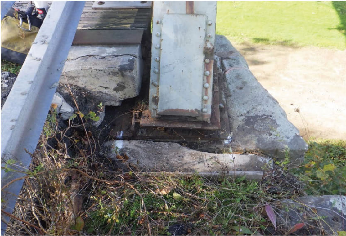
5. Far Abutment bearing shifted to left on the Left Truss.
