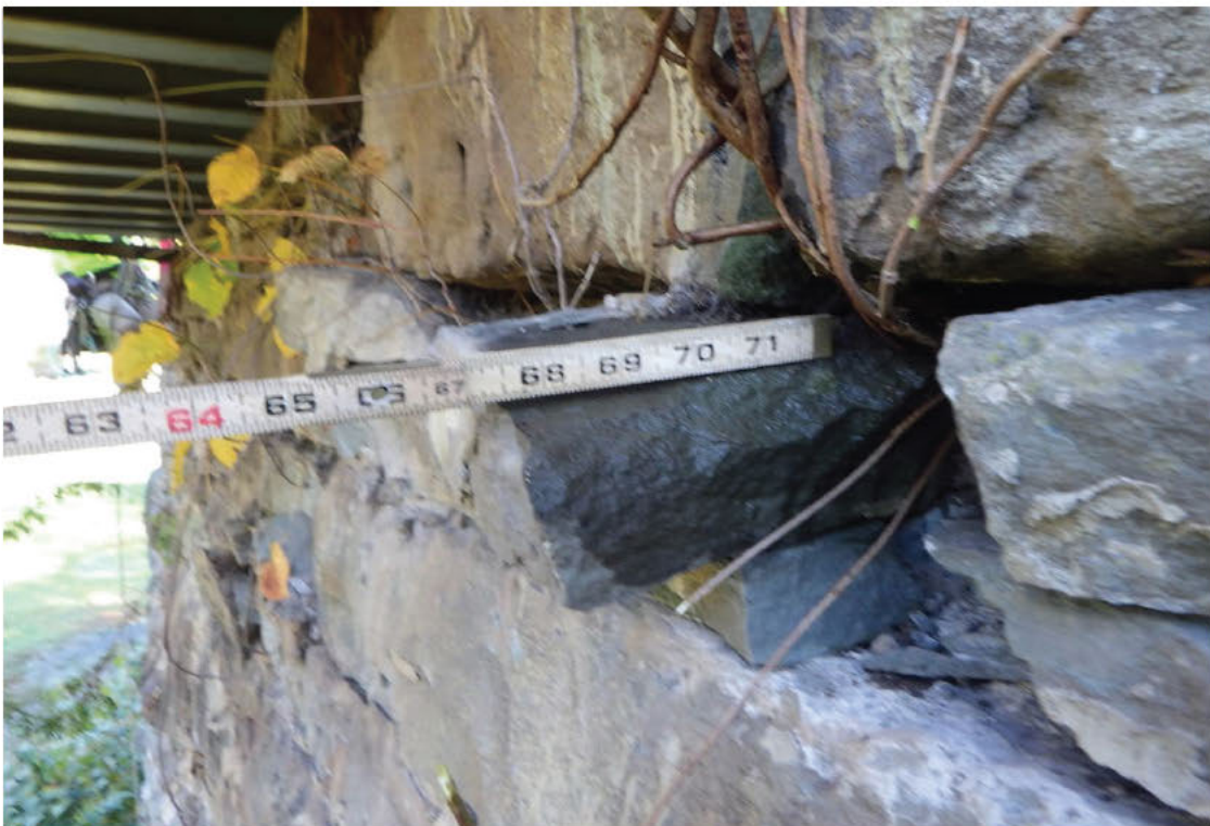
14. Close-up of previous photo showing displaced stone.
