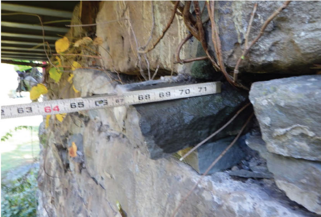
111. Displaced stone and missing mortar at the Far Abutment.
