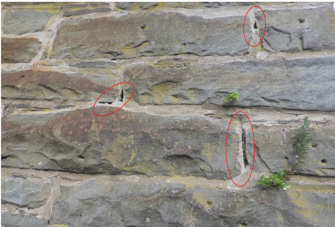
104. Close-up of deteriorated mortar on the near face of Pier 1.
