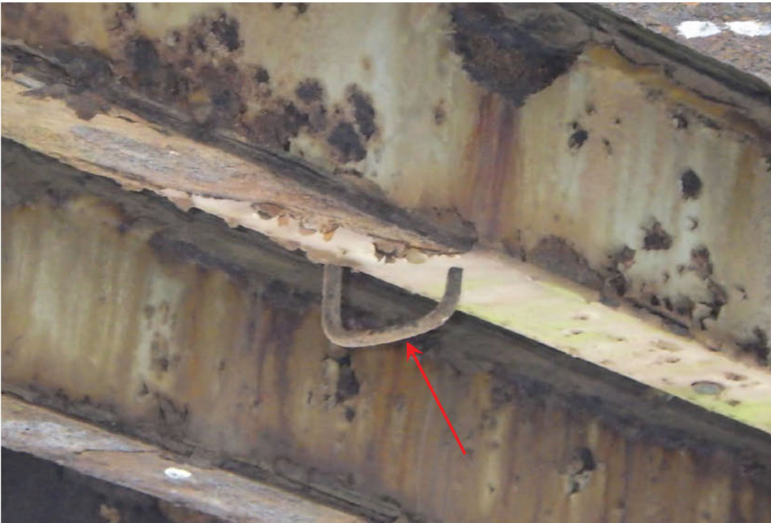
60. Loose "J" hook not engaging stringer bottom flange, Stringer Bay 5 in Span 2.
