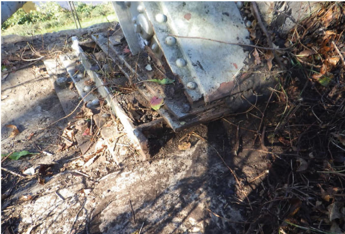
84. Superstructure shifted left with exposed rollers at the Right Truss bearing on the Far Abutment.
