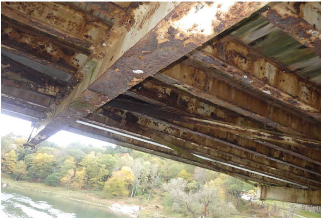
48. Typical condition of floorbeam bottom flange, FB 3 in Span 2, looking right.
