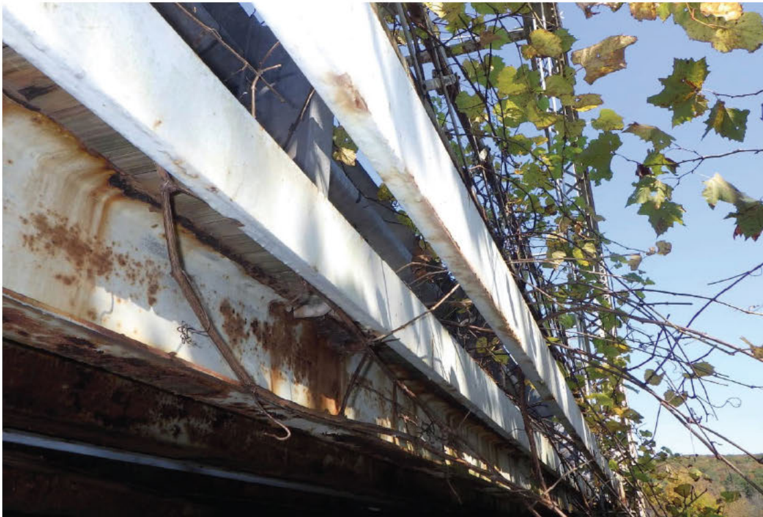
30. Bottom chord with vegetation growth, L0-L1, Right Truss in Span 1.
