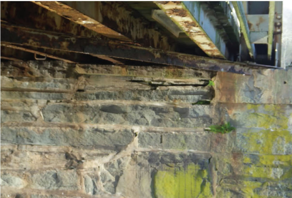
106. Area of missing mortar on the far face of Pier 1.
