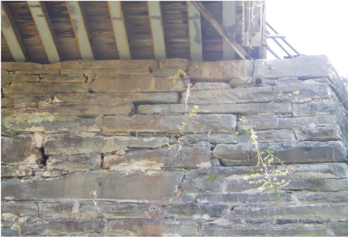
13. Area of loose/displaced stones and missing mortar at right end of the Far Abutment.
