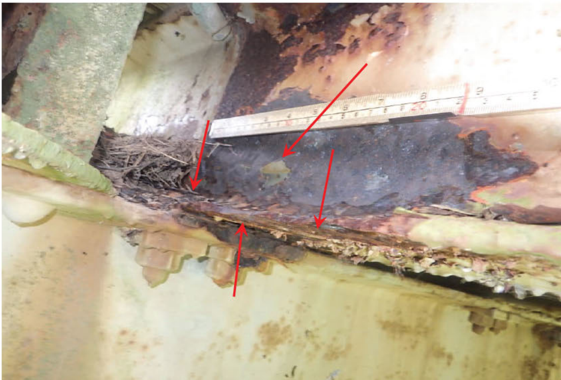
56. Section loss to web and bottom flange of Stringer 11 at Floorbeam 8 in Span 2.
