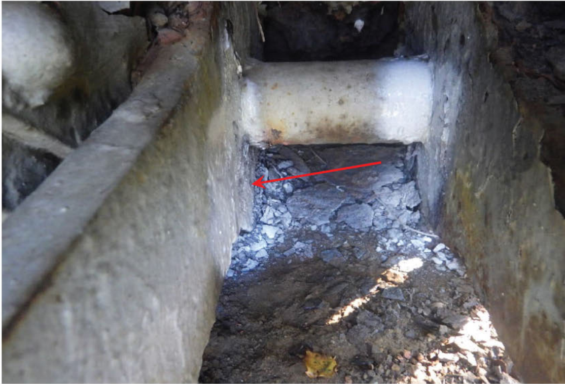
27. Severe corrosion to L11-L12 at L12, Right Truss in Span 2.
