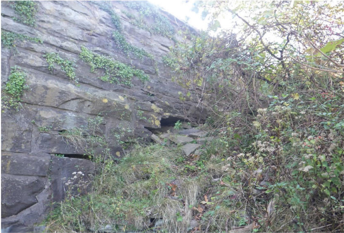
99. Missing stones with void along the base of the Near Left wingwall.
