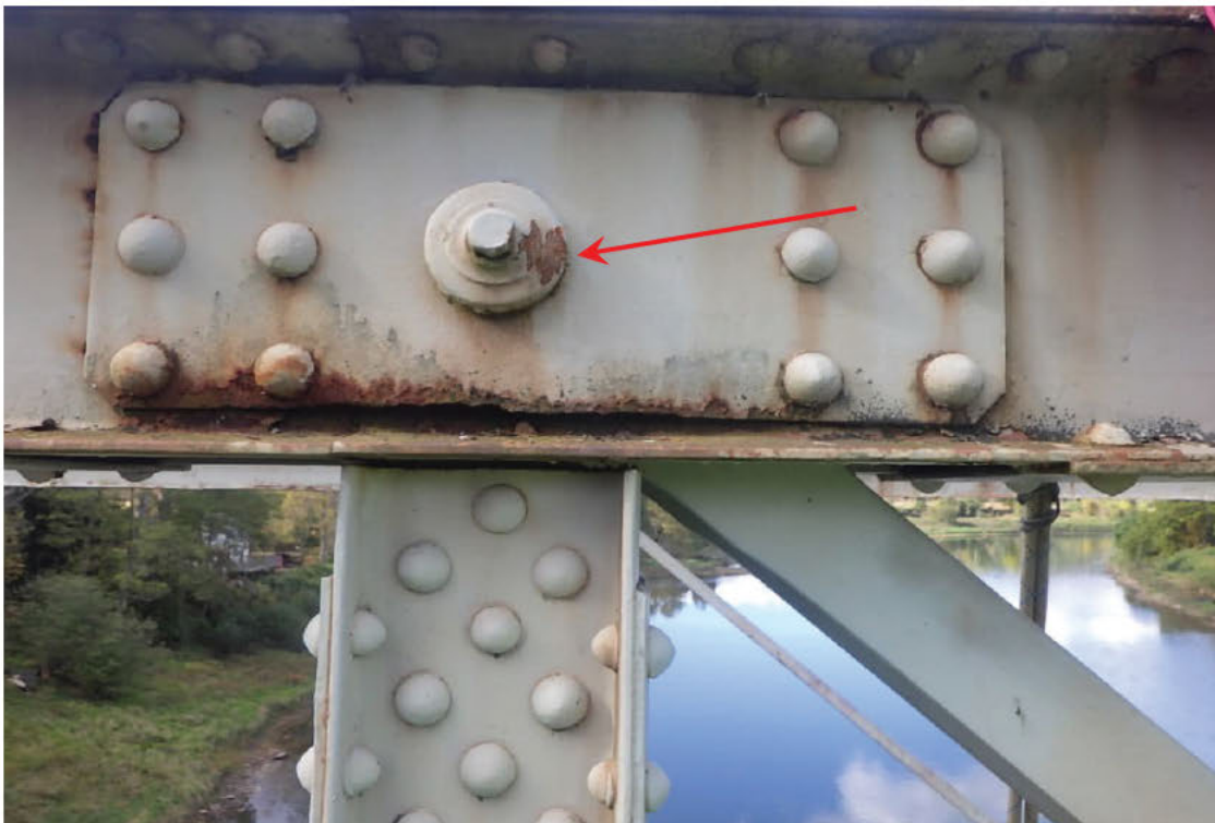
38. Cracked outboard pin cap at U4, Right Truss, Span 1.
