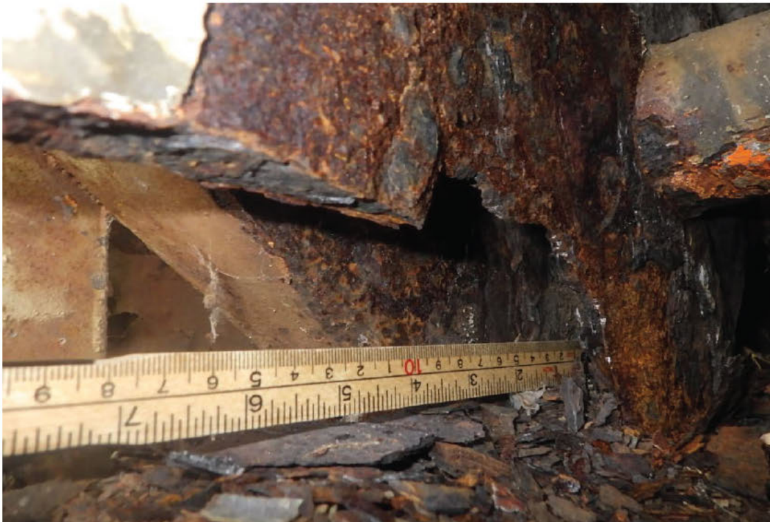
26. Close-up of previous photo showing section loss to eyebar head.
