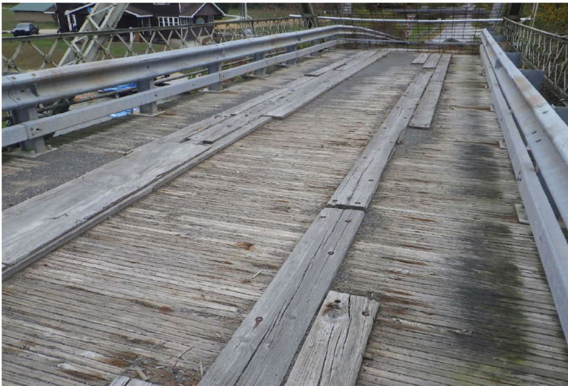
14. Typical missing running planks in Span 2.
