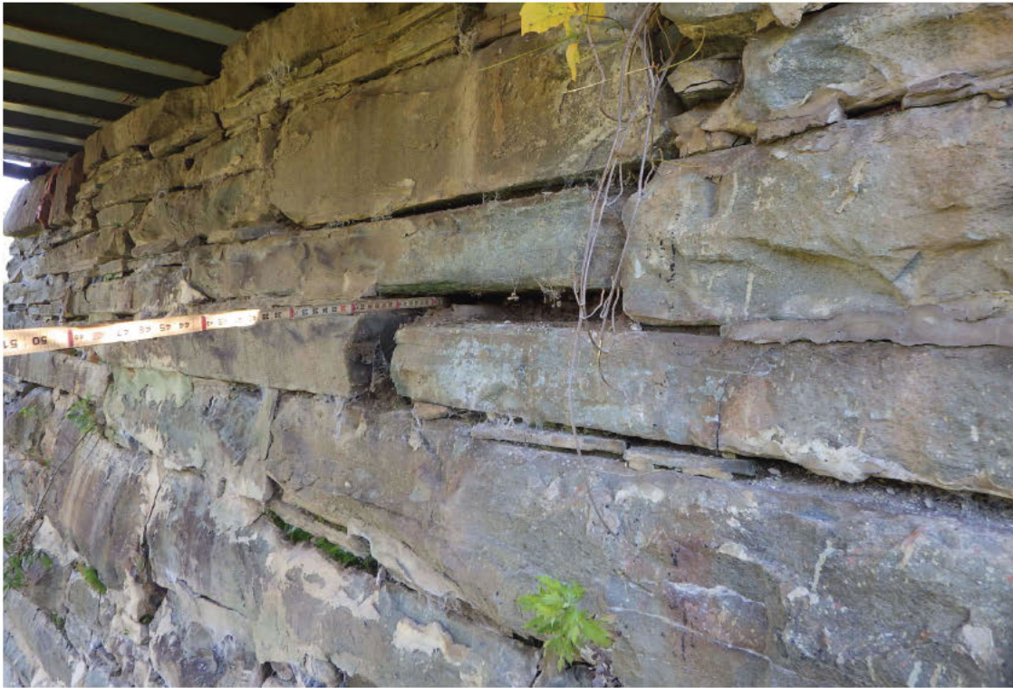
15. Deep void and loose stones on the right side of the Far Abutment.
