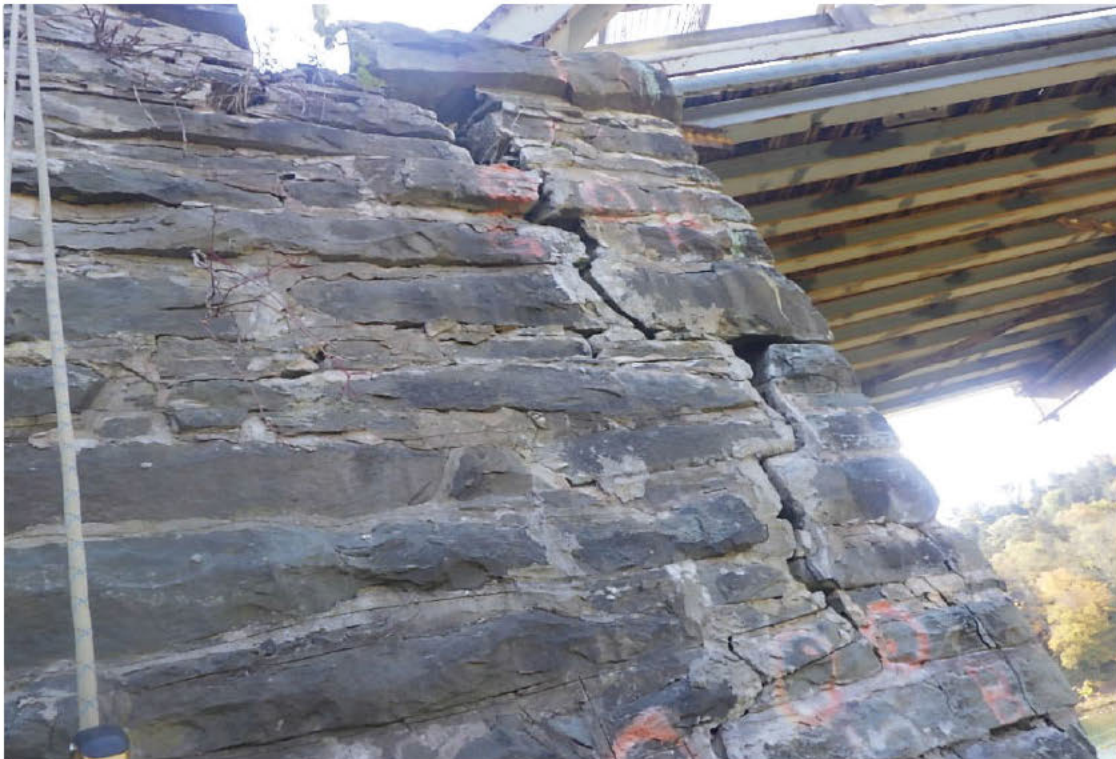
18. Wide crack with loose stones and missing mortar in the Far Left Wingwall.
