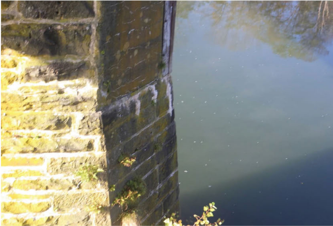
107. Cracks with efflorescence on the left nose of Pier 1.
