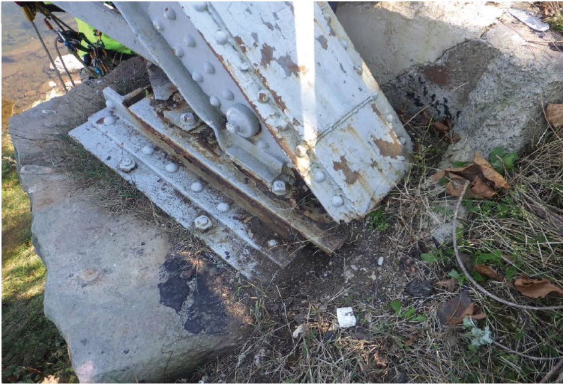
1. Overexpanded Left Truss Bearing at Near Abutment.
