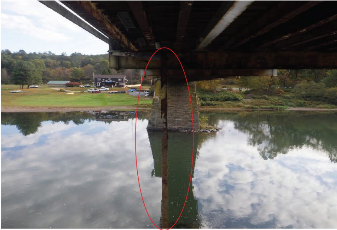
69. Disconnected left lower lateral brace, Bay 4 in Span 1. (Removed during inspection)
