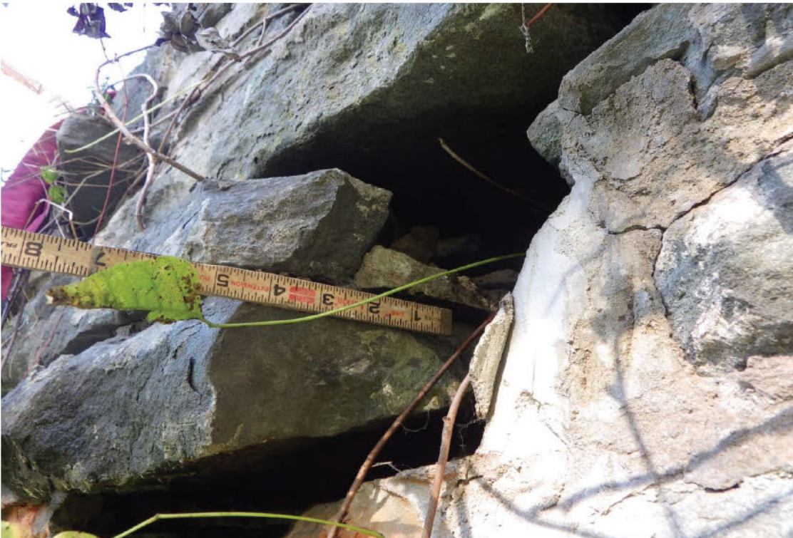
124. Displaced stones above monitoring point A-B at the Far Right wingwall.
