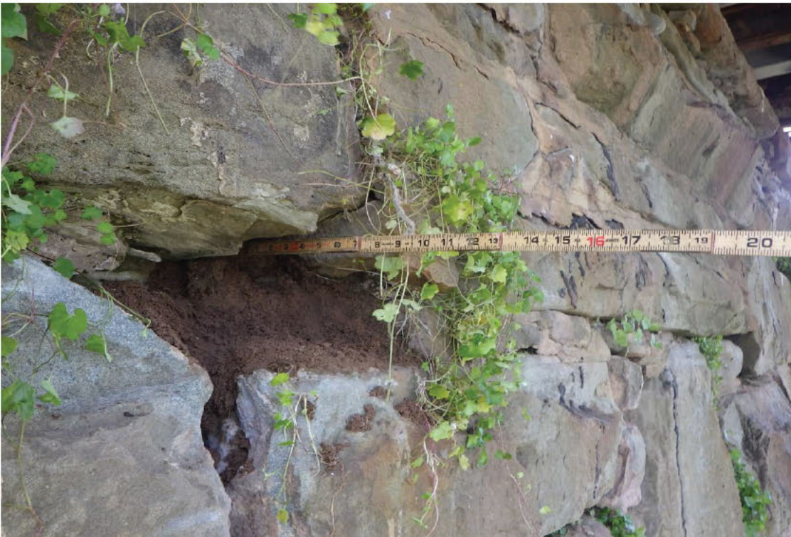
94. Missing stone below Stringer 10 at the Near Abutment.
