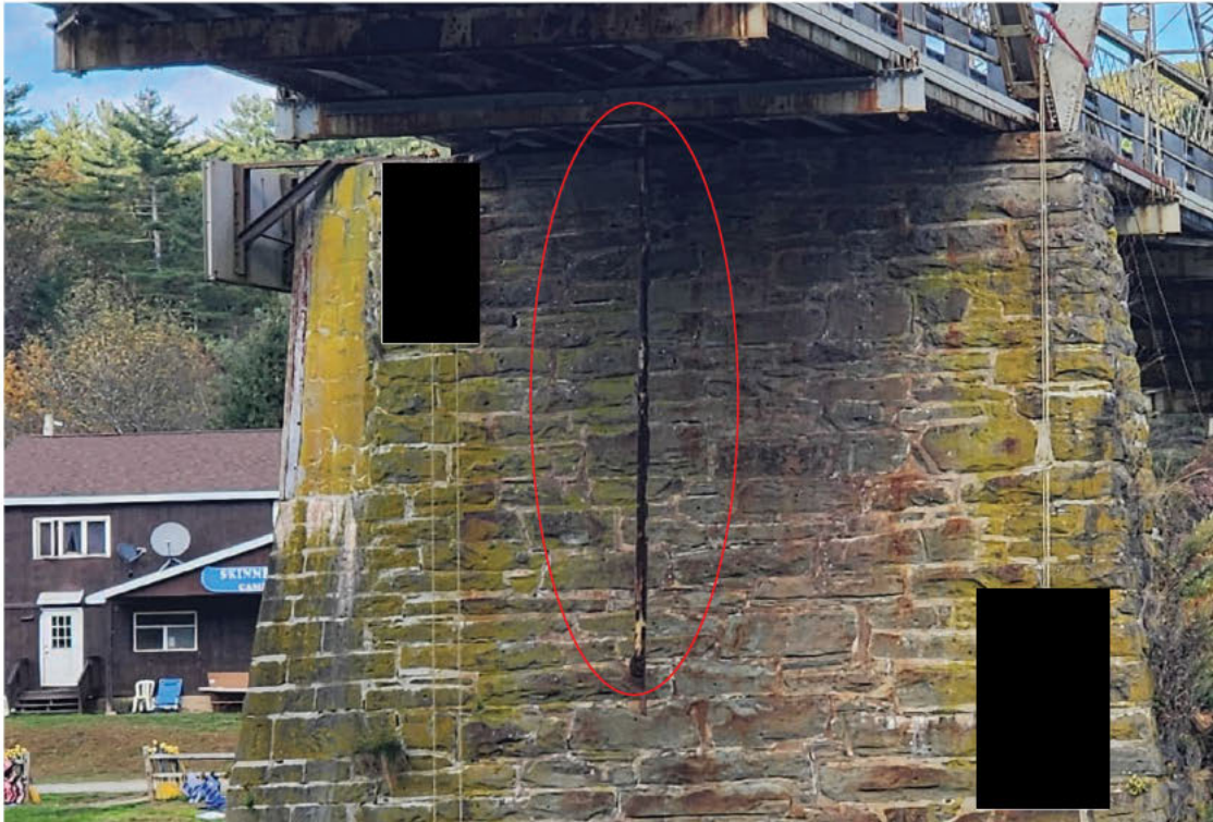
67. Disconnected right lower lateral brace, Bay 12 in Span 1. (Removed during inspection)
