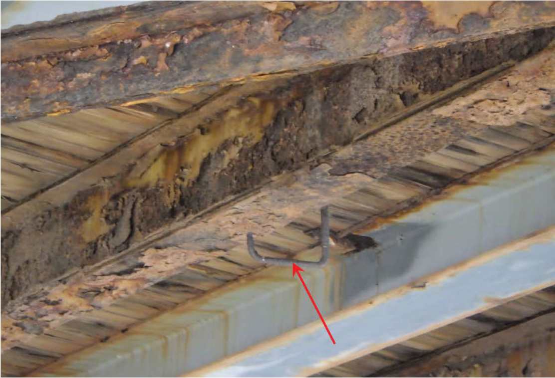
59. Loose "J" hook not engaging stringer bottom flange, Stringer Bay 1 in Span 1.
