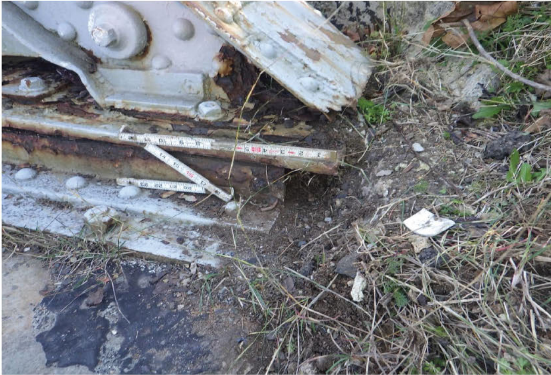
73. Left Truss bearing sole plate overhanging nested rollers at the Near Abutment.
