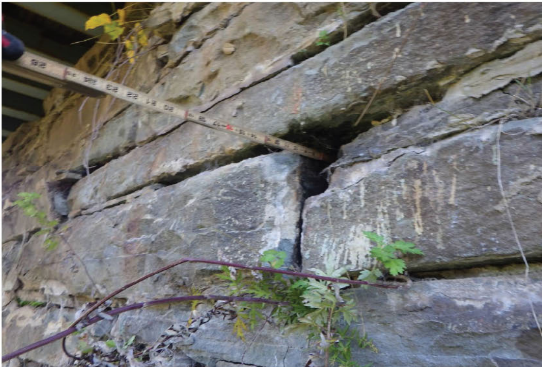
112. Missing mortar and deep voids at the Far Abutment.
