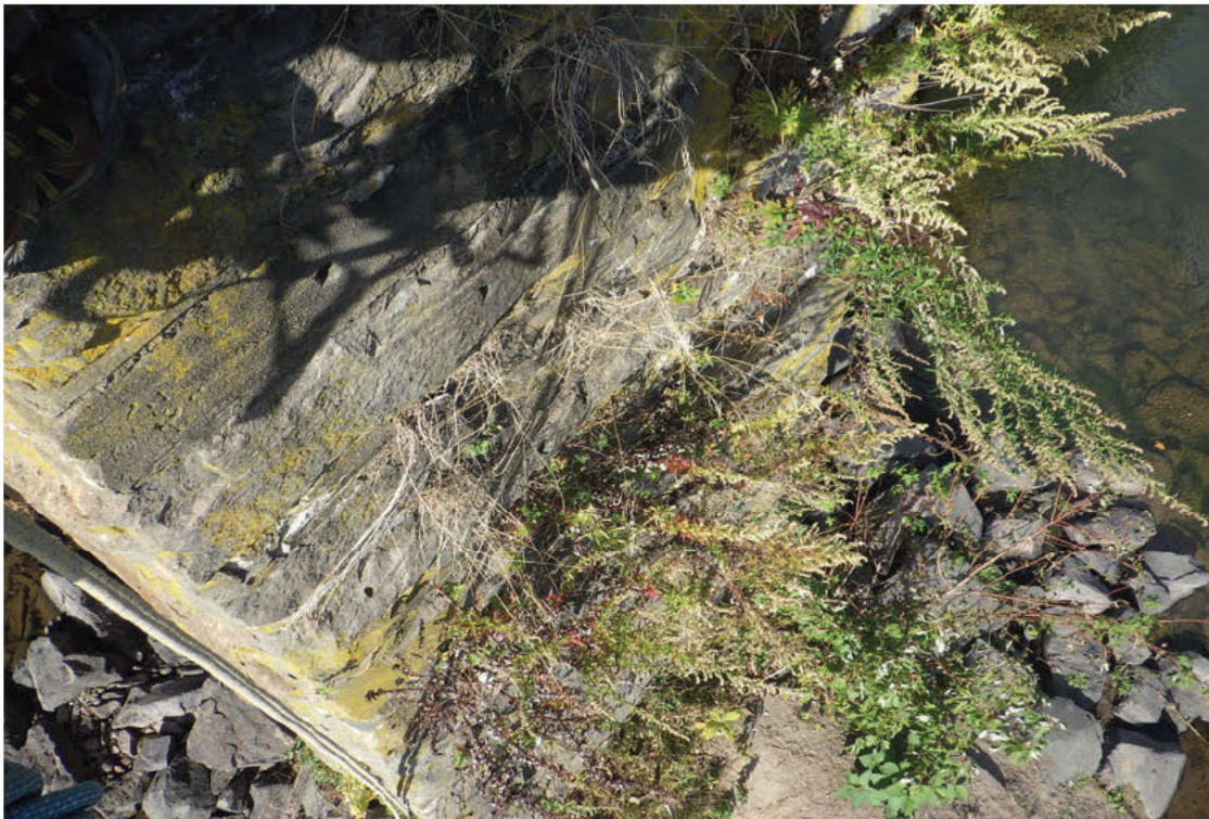
108. Vegetation growth on the right nose of Pier 1.
