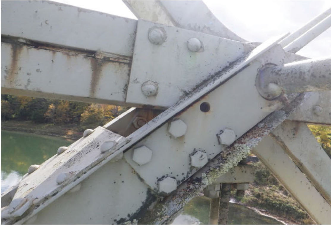
33. Mis-drilled hole, M7-L8 at M7, Right Truss, Span 1.
