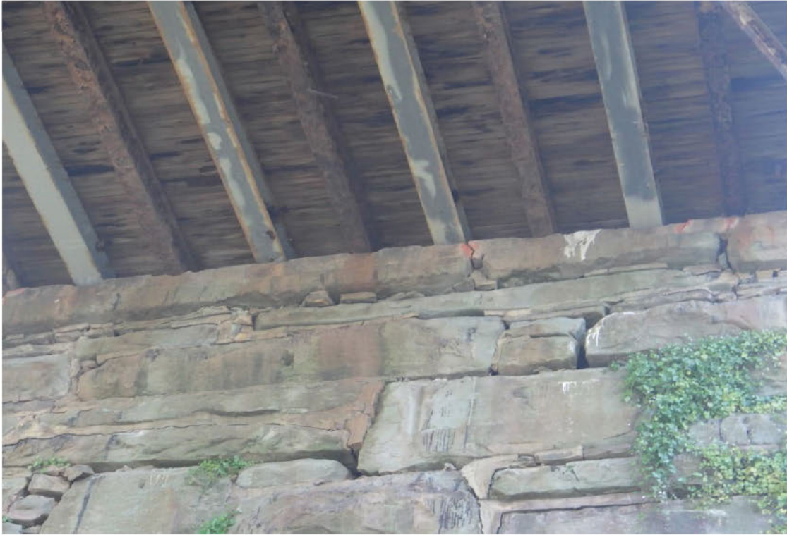
11. Area of loose stones and missing mortar at left end of the Near Abutment.
