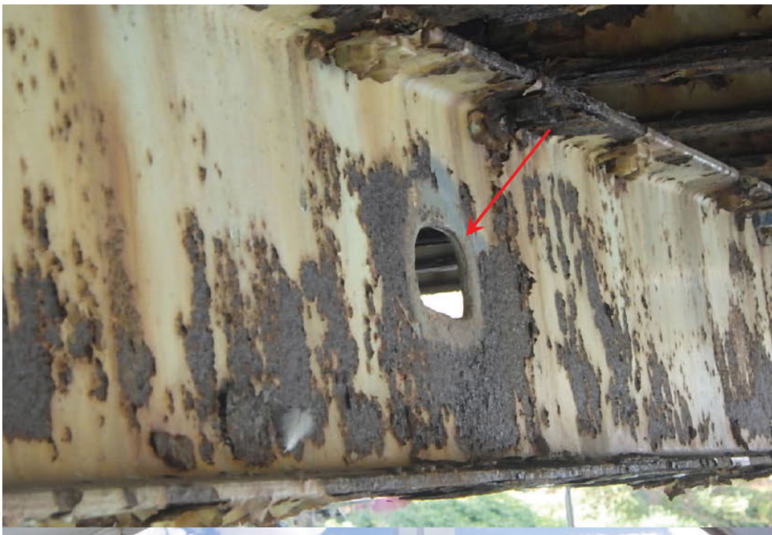
52. Flame cut hole in web of Floorbeam 4 in Span 1.
