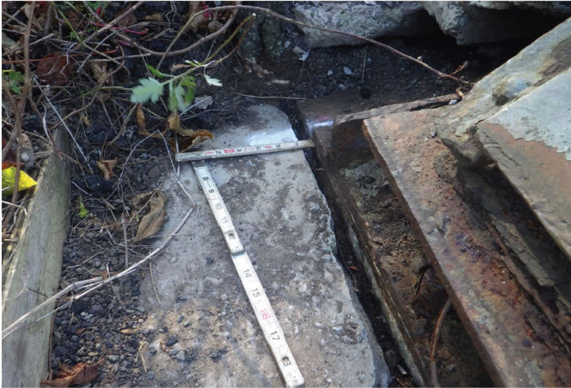
115. Separation of repair and left truss bearing at the Far Abutment.
