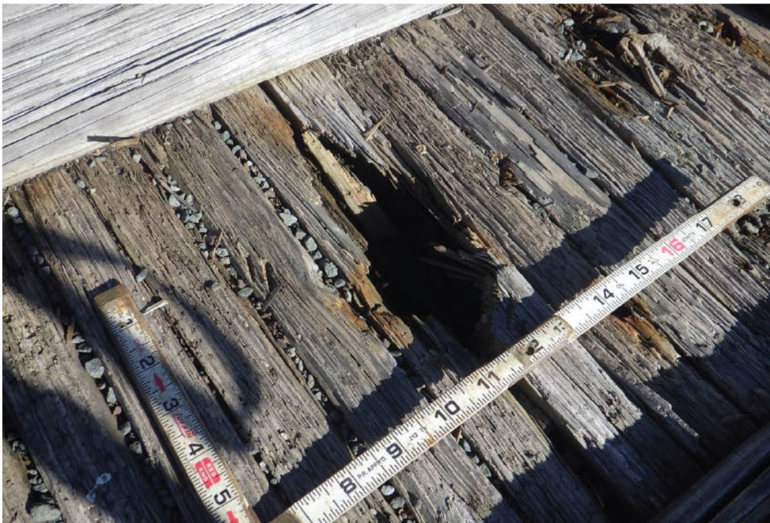
16. Close-up of previous photo showing severe decay to deck boards.
