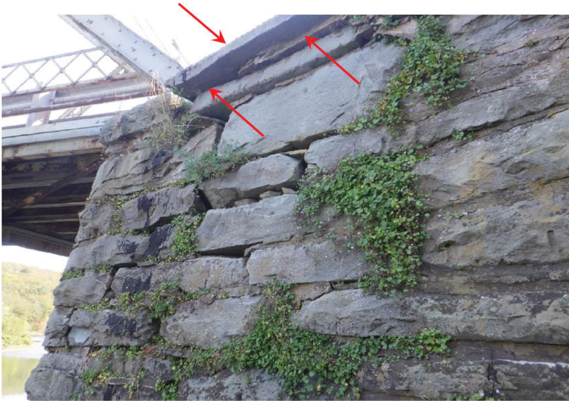
97. Shifted cap stone at the Near Left wingwall.
