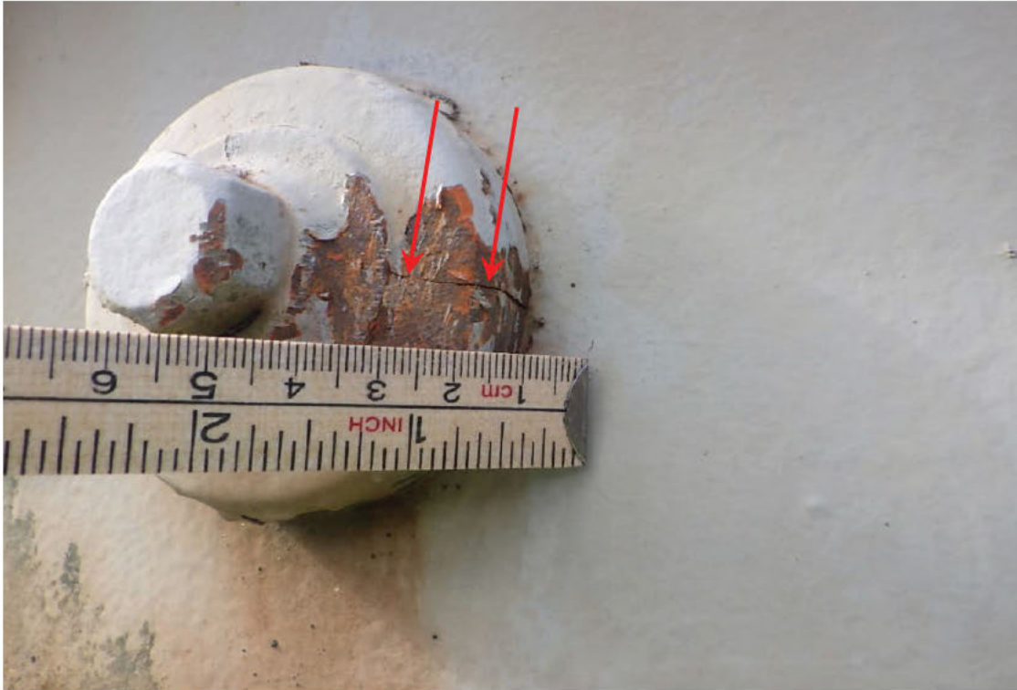
39. Cracked outboard pin cap at U4, Right Truss, Span 1.
