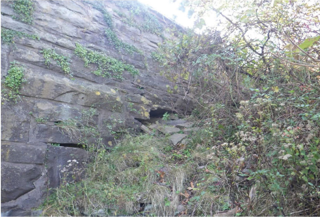
9. Near Left wingwall with large void due to missing stones.
