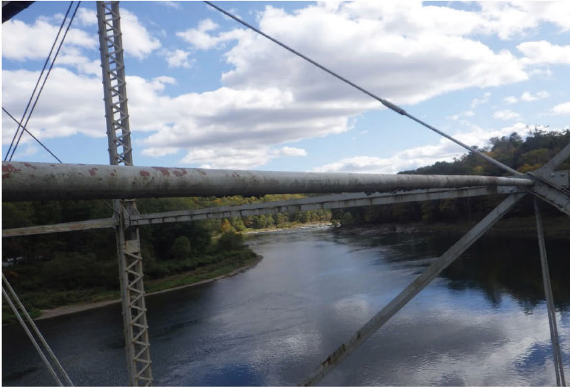
43. Collision damage to horizontal strut of sway bracing, M5 in Span 1, looking right.
