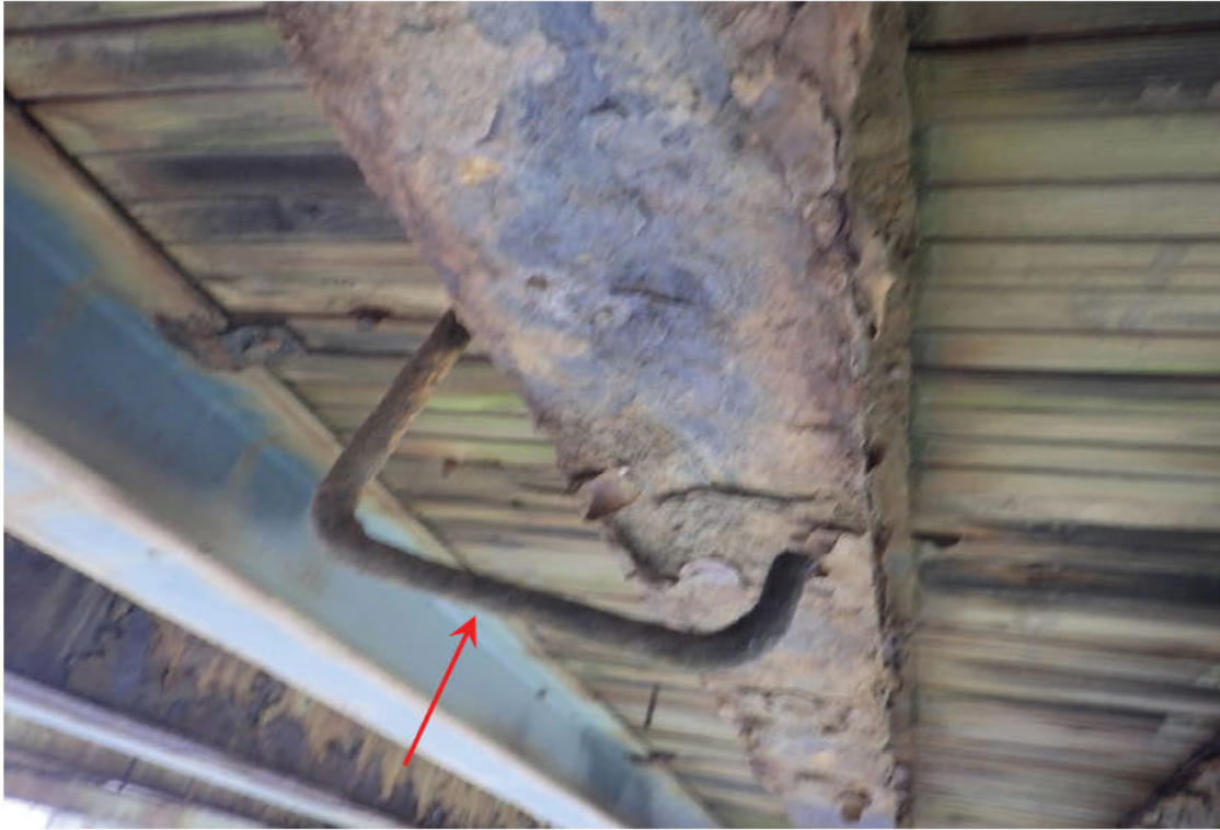
61. Loose "J" hook not engaging stringer bottom flange, Stringer Bay 10 in Span 1.
