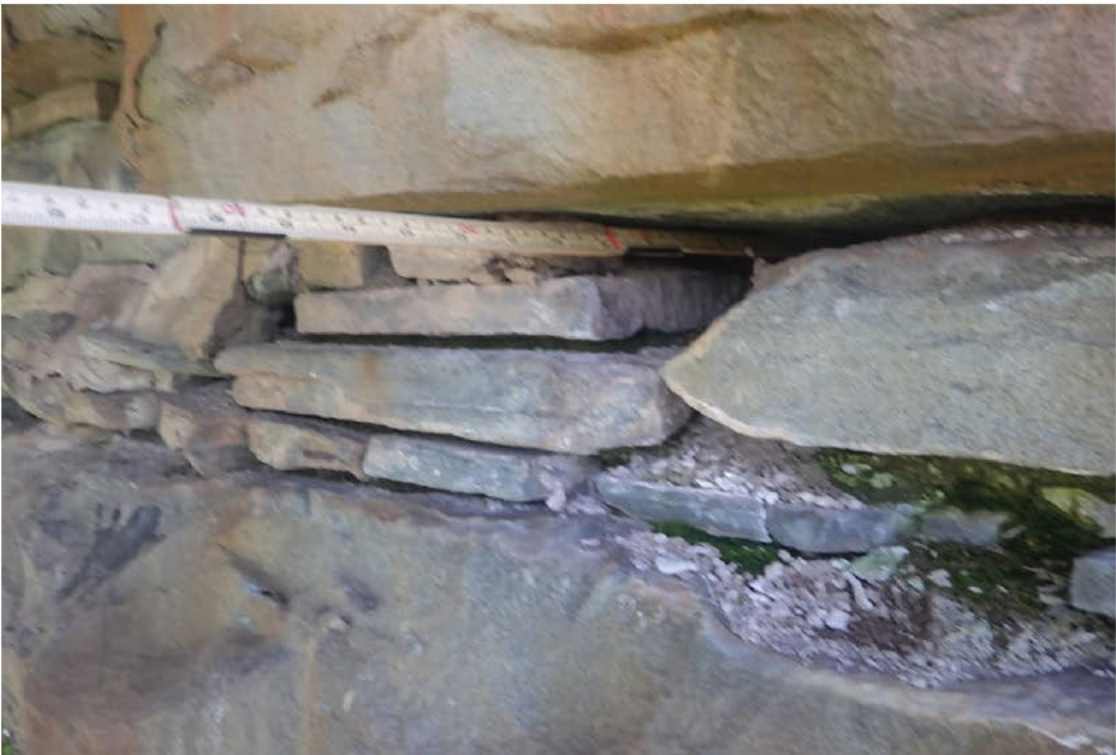
90. Close-up of previous photo showing deep voids in mortar joints.
