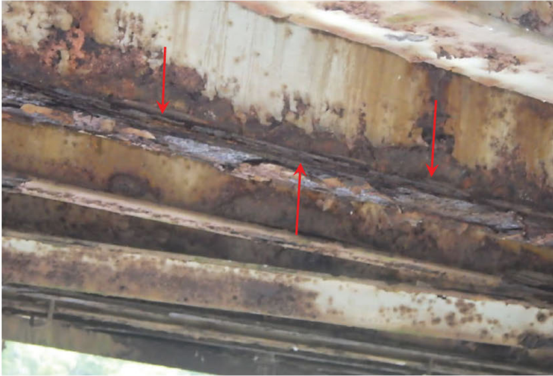
55. Section loss to bottom flange of Stringer 8 in Floorbeam Bay 4 of Span 2.
