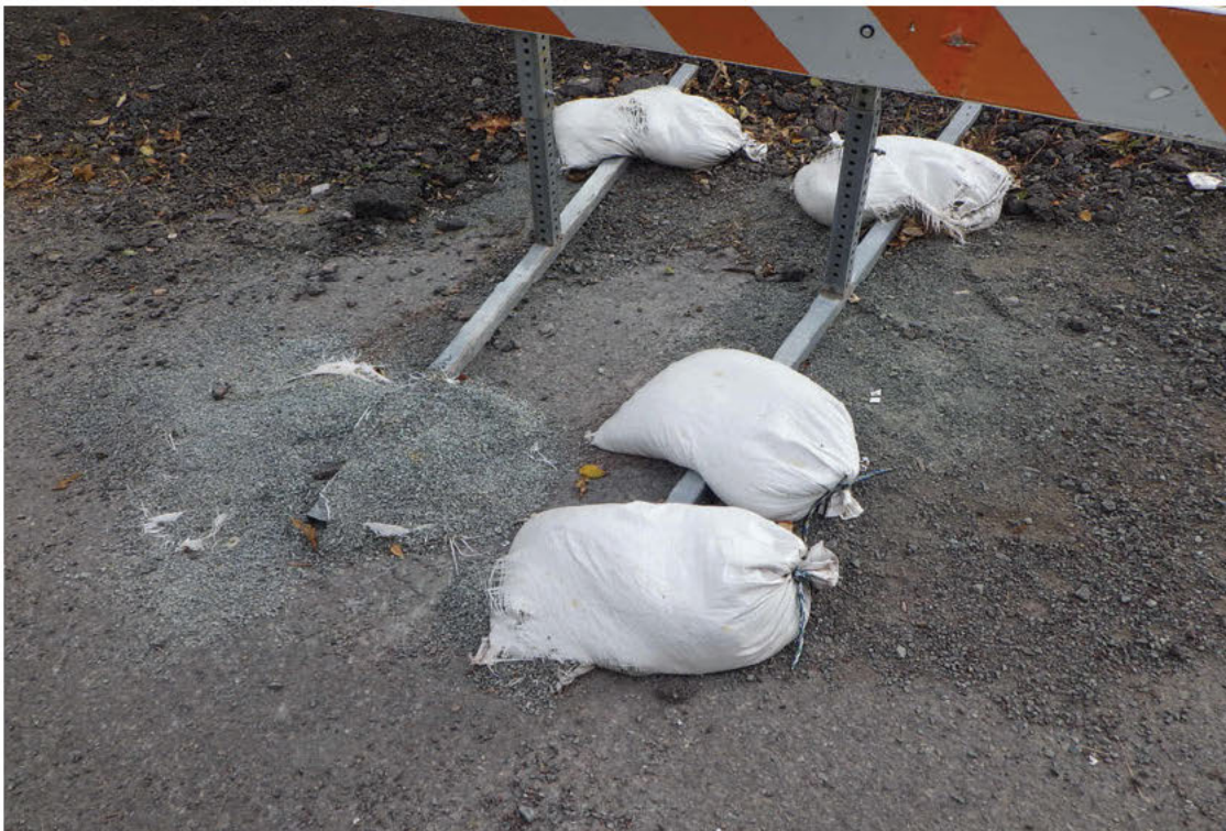
8. Damaged gravel bag at the near approach.
