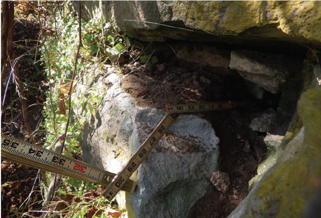
101. Missing stone with void in the Near Right wingwall.
