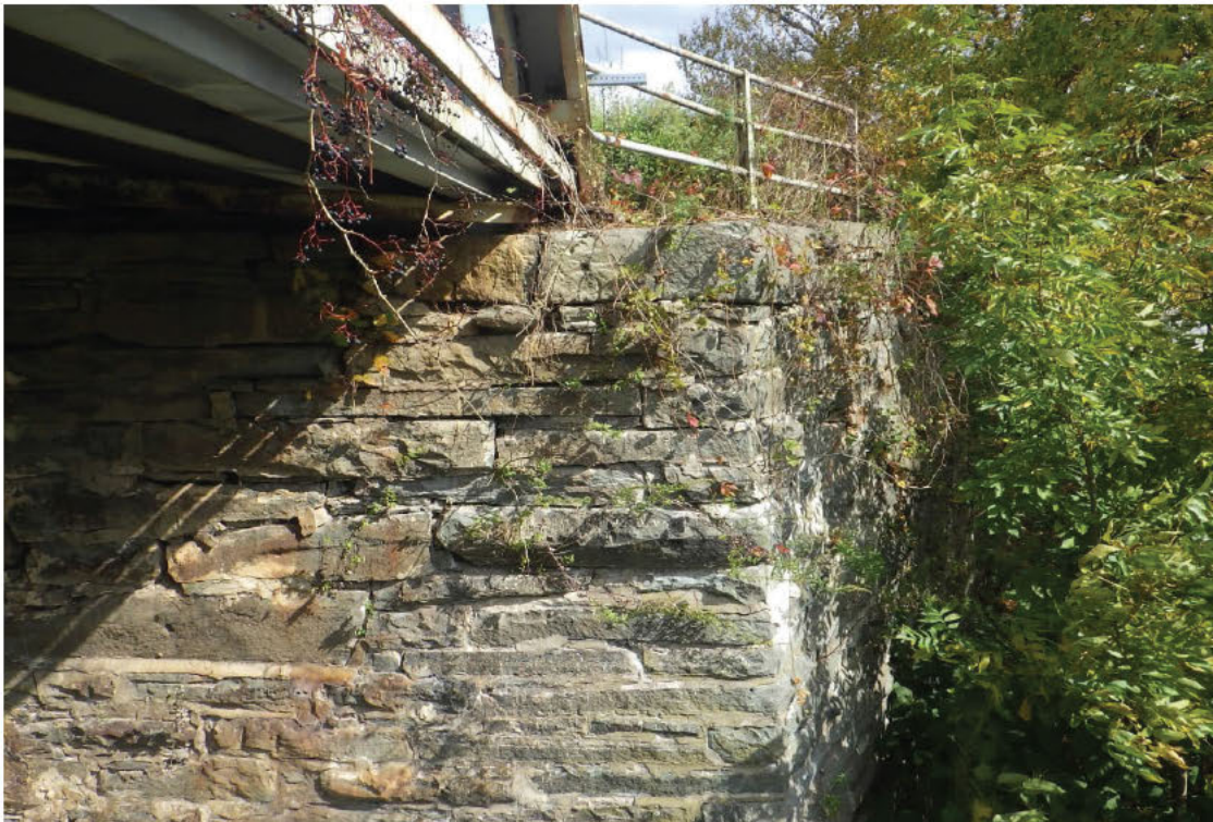
110. Missing mortar and displaced stones on the right side of the Far Abutment.
