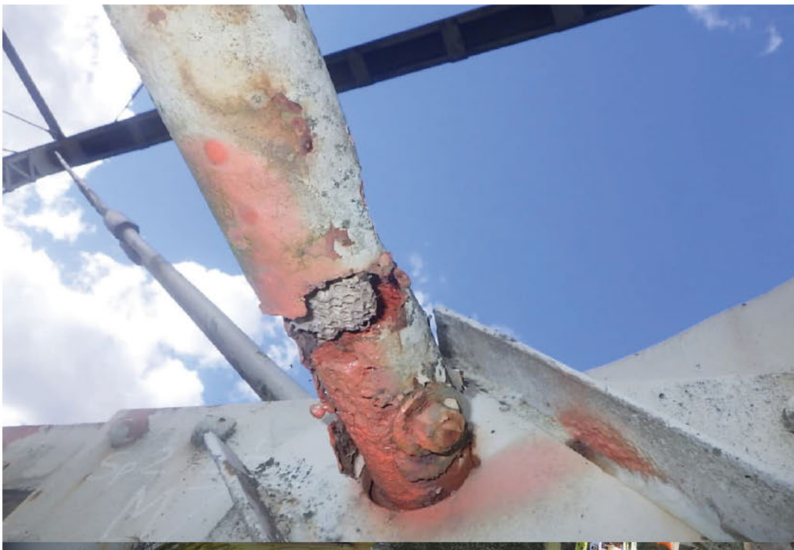
44. 100% section loss to horizontal strut of sway bracing at M7, Left Truss in Span 2.
