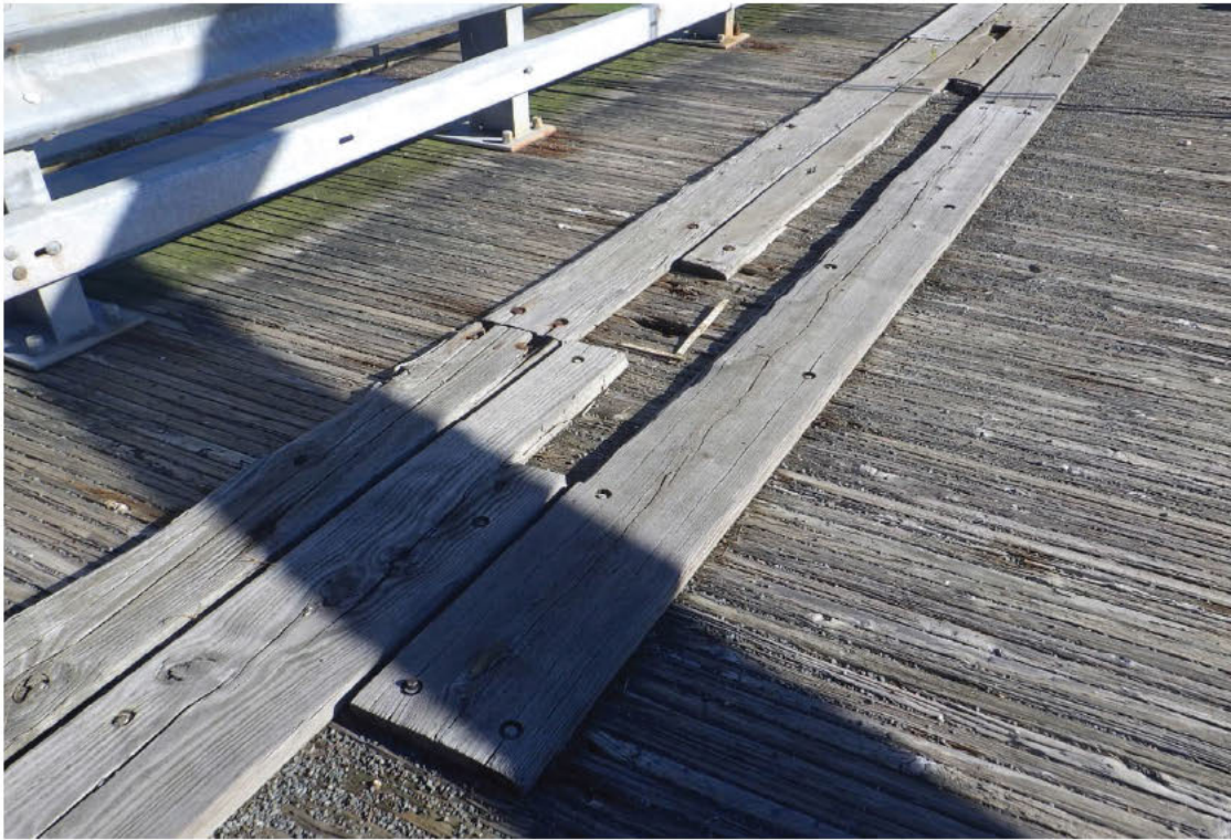
15. Missing running planks with severe decay to below to laminated deck boards in Span 2.
