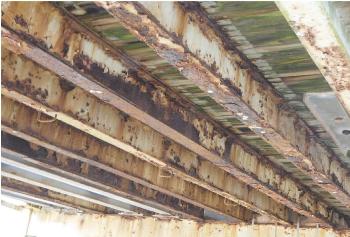
54. Typical stringer condition in Span 2 between Floorbeam 4 & 5, looking back.
