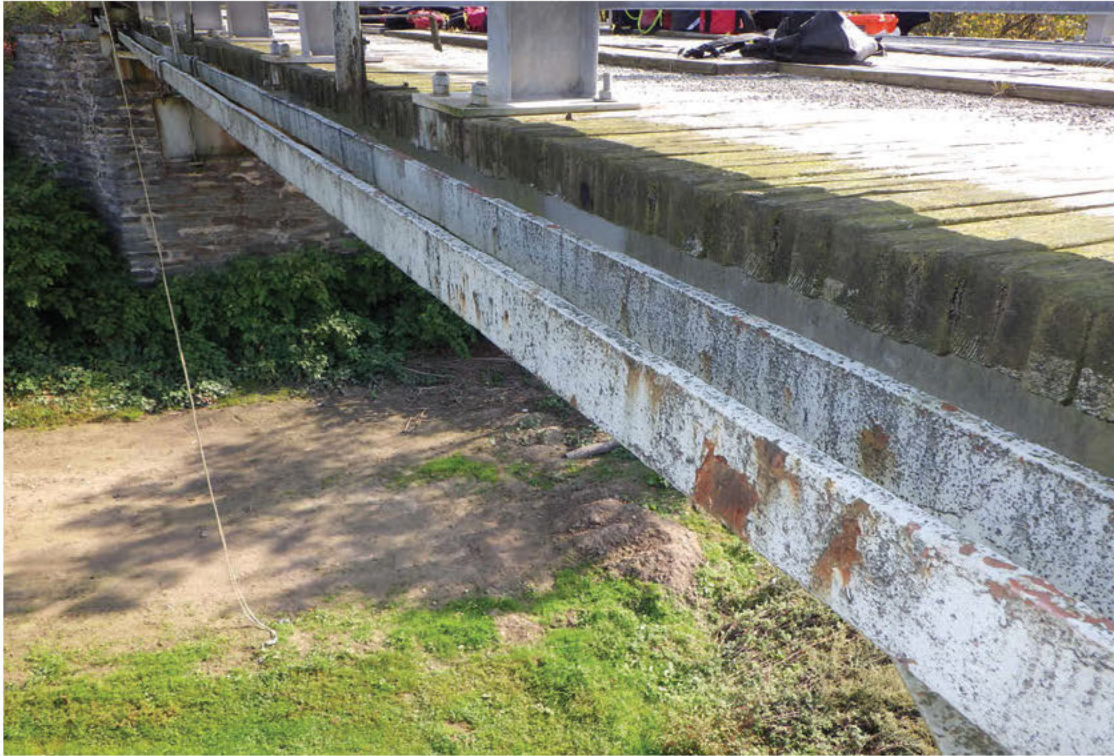
21. Typical bottom chord condition, L8-L9, Left Truss in Span 2, looking ahead.
