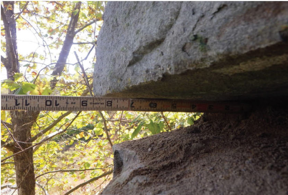
92. Close-up of previous photo showing undermining of the capstone.
