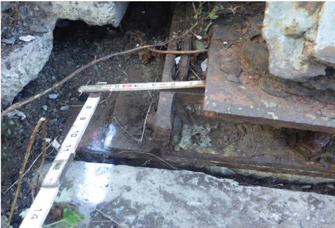
6. Close-up of previous photo showing exposed rollers.
