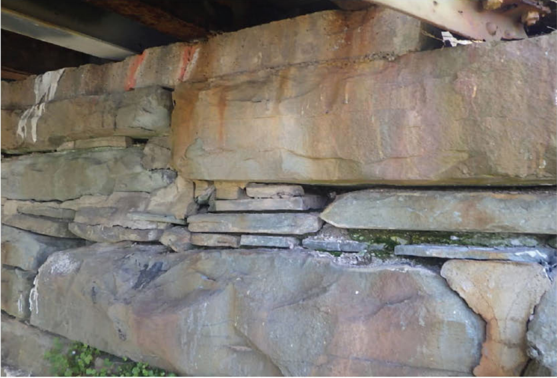
89. Area of deteriorated mortar and loose stones below Stringer 4 to Left Truss, Near Abutment.
