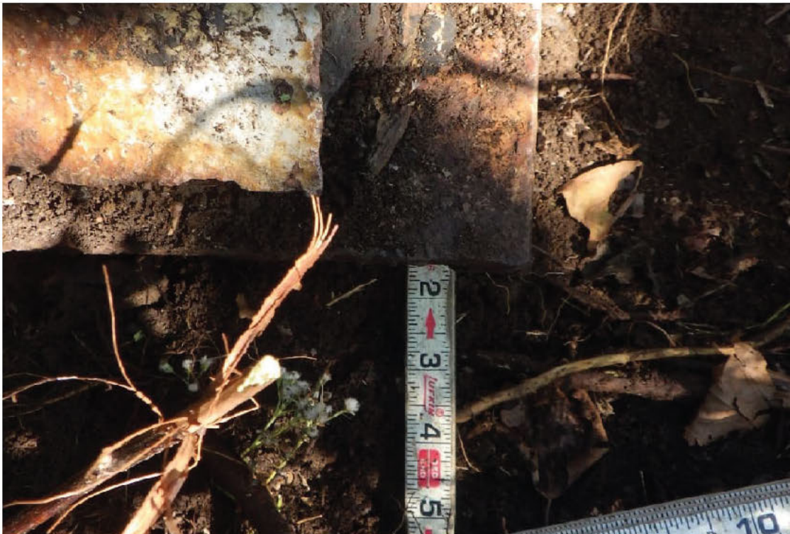
76. Close-up of previous photo, showing sole plate overhanging the nested roller bearings.
