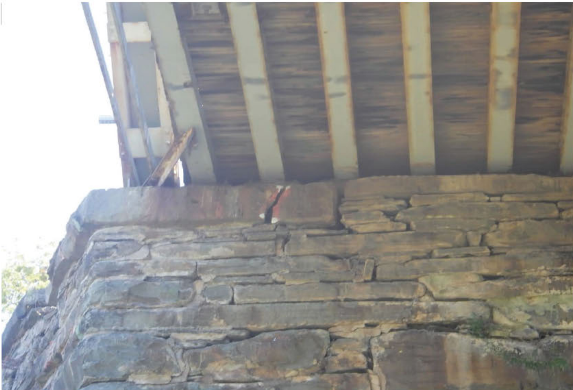
12. Area of loose stones and missing mortar at left end of the Far Abutment.
