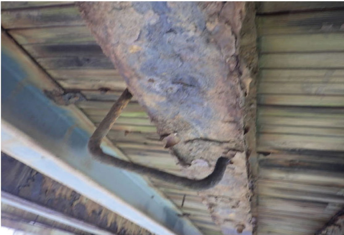
22. Loose deck "J" hook in Span 2, between FB 9 & 10.
