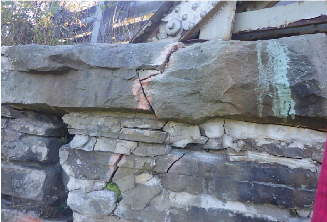
113. Fractured capstone on the Left side of the Far Abutment.
