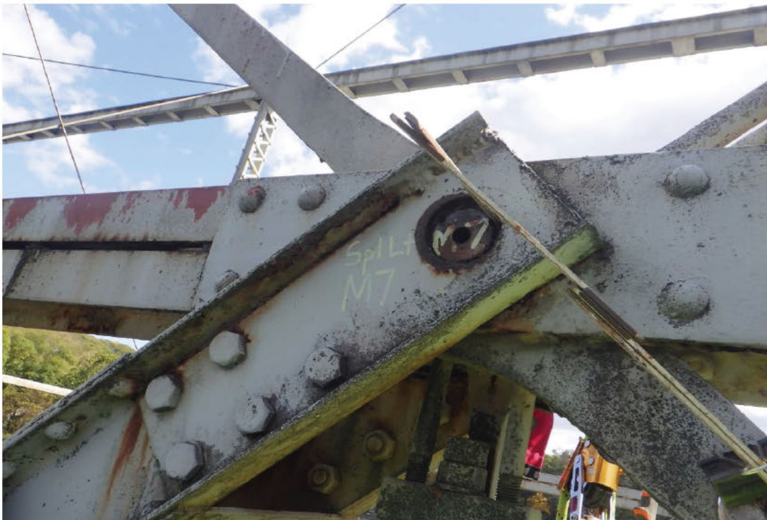
34. Missing pin cap for M7-L8 at M7, Left Truss, Span 1.
