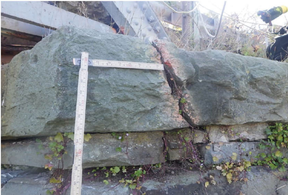
96. Fractured cap stone at the left end of the Near Abutment.
