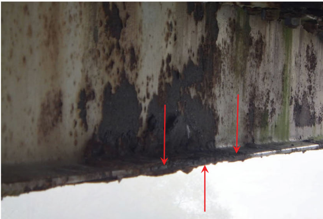
50. Section loss to bottom flange of Floorbeam 5 in Span 2, looking right.
