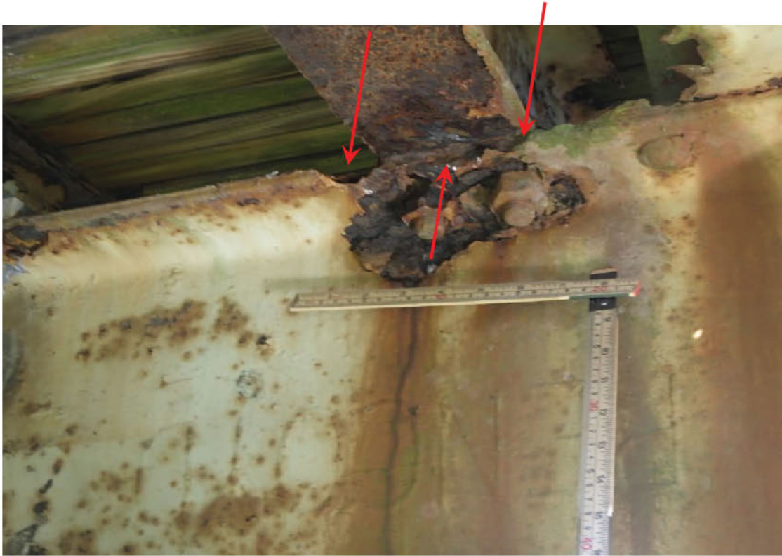
51. Section loss to top flange of Floorbeam 10 in Span 2, adjacent to Stringer 11.
