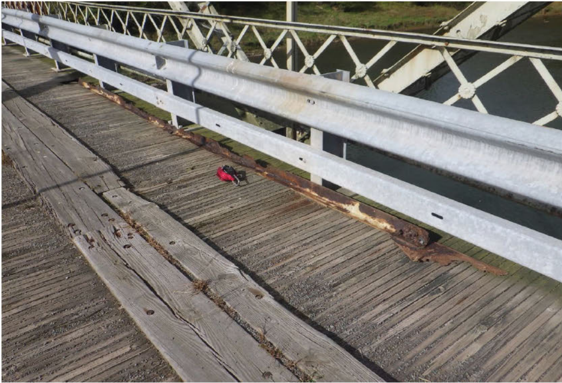
21. Loose right lower lateral brace member removed and left on the top of deck, Span 1 between FB 11 & 12.
