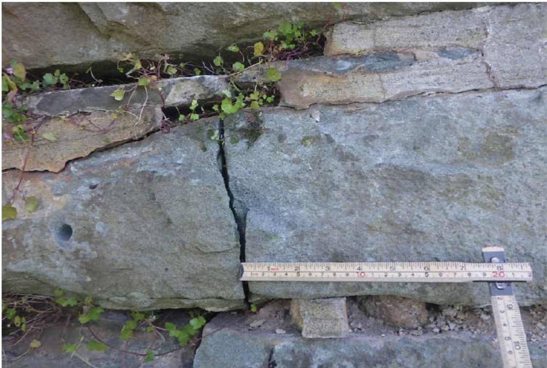
88. Fractured stone in 5th coarse below Left Truss a the Near Abutment.
