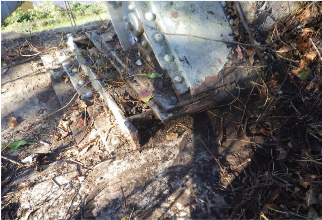
3. Far Abutment bearing shifted to left on the Right Truss.
