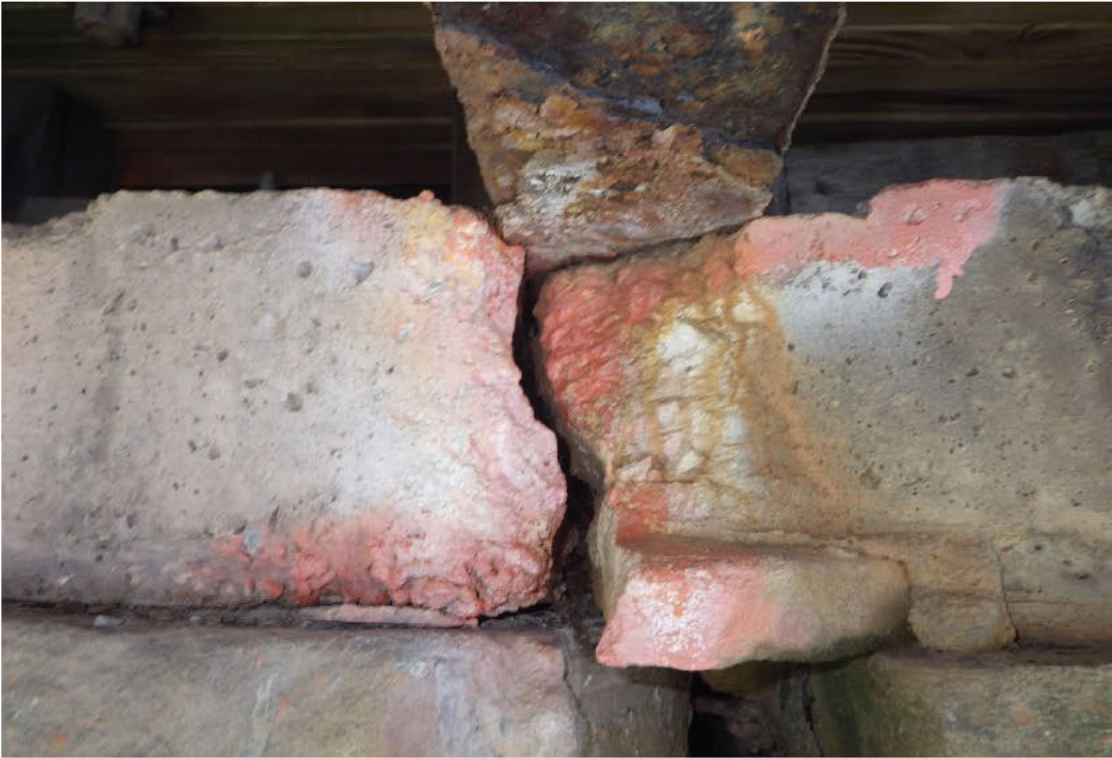
93. Fractured cap stone below Stringer 10 at the Near Abutment.
