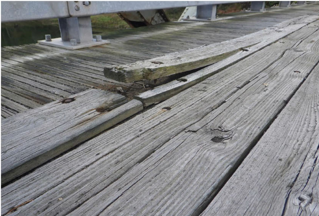
12. Typical warped running plank with missing fasteners.
