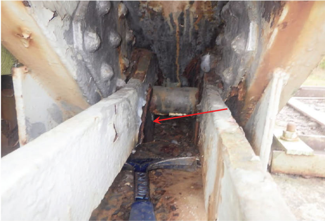
25. Severe corrosion to L0-L1 at L0, Left Truss in Span 2.
