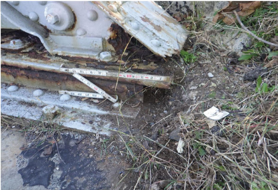
2. Close-up of previous Photo showing sole plate overhanging nested rollers.
