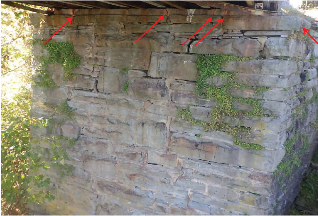
87. Several fractured cap stones along the top of the Near Abutment.
