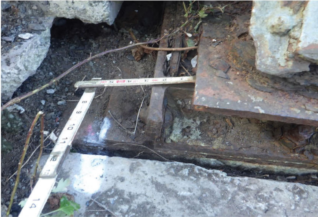
81. Sole plate shifted left on the left truss bearing at the Far Abutment.
