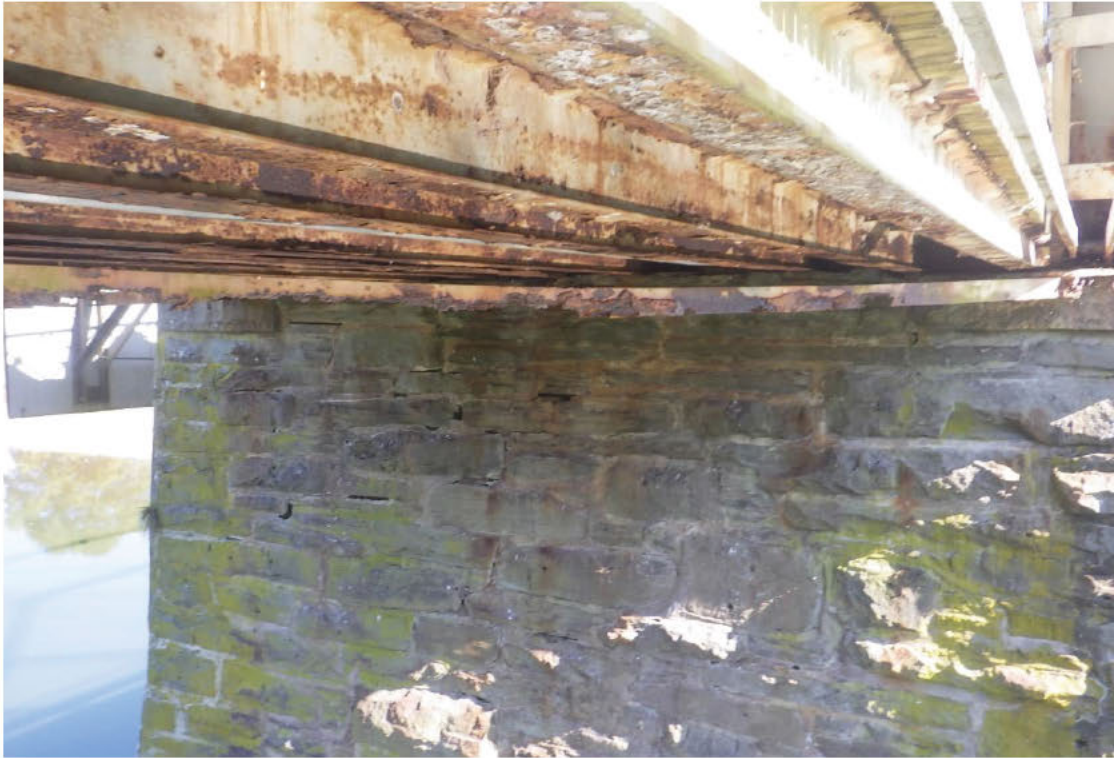
103. Areas of missing mortar along the top of the near face of Pier 1.
