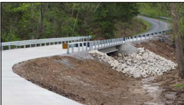
The new Spring Fork Bridge is seen Tuesday. The Missouri Department of Transportation unexpectedly closed the unsafe bridge last year. Pettis County funded a new $500,000 bridge out of the reserve fund. PHOTO BY CHRIS HOWELL | DEMOCRAT
