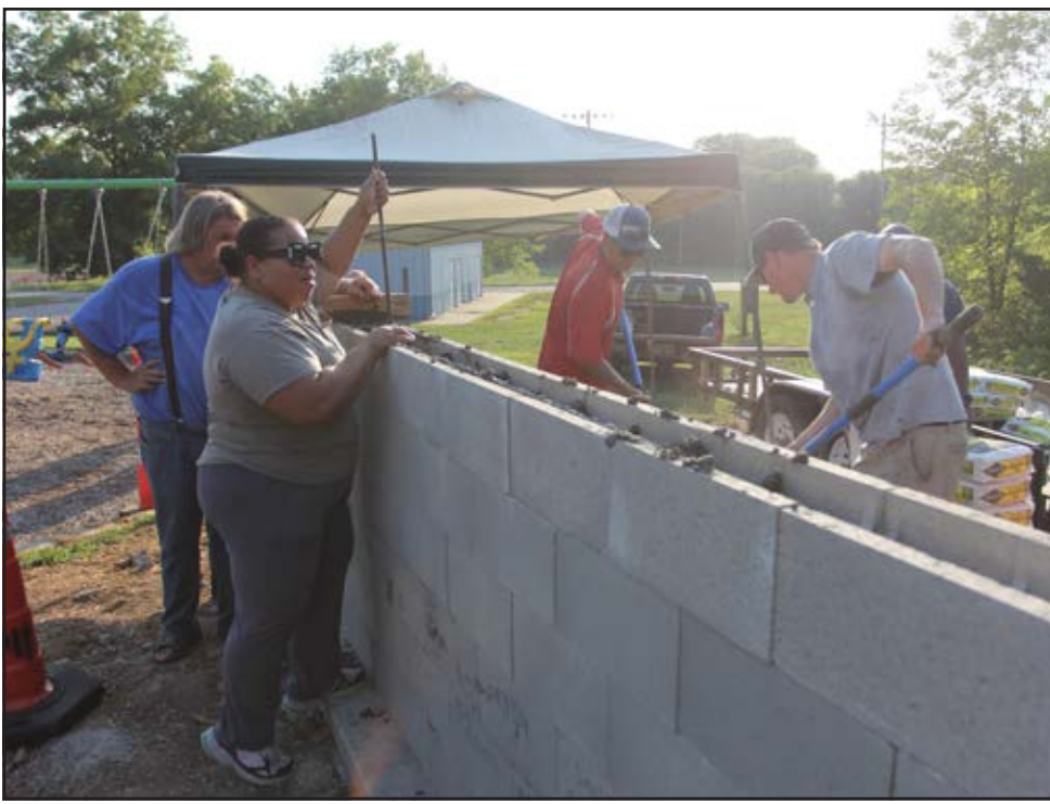
Parks and Recreation Board President Erica Collins helps to fill the wall with concrete during a community build Thursday, Aug. 25, at the Inclusive Playground. Collins and Scott Holmberg placed a tea bag and coffee beans, respectively, inside the wall as symbols of the partnership between the Parks and Recreation Department and the Johnson County Board of Services.
