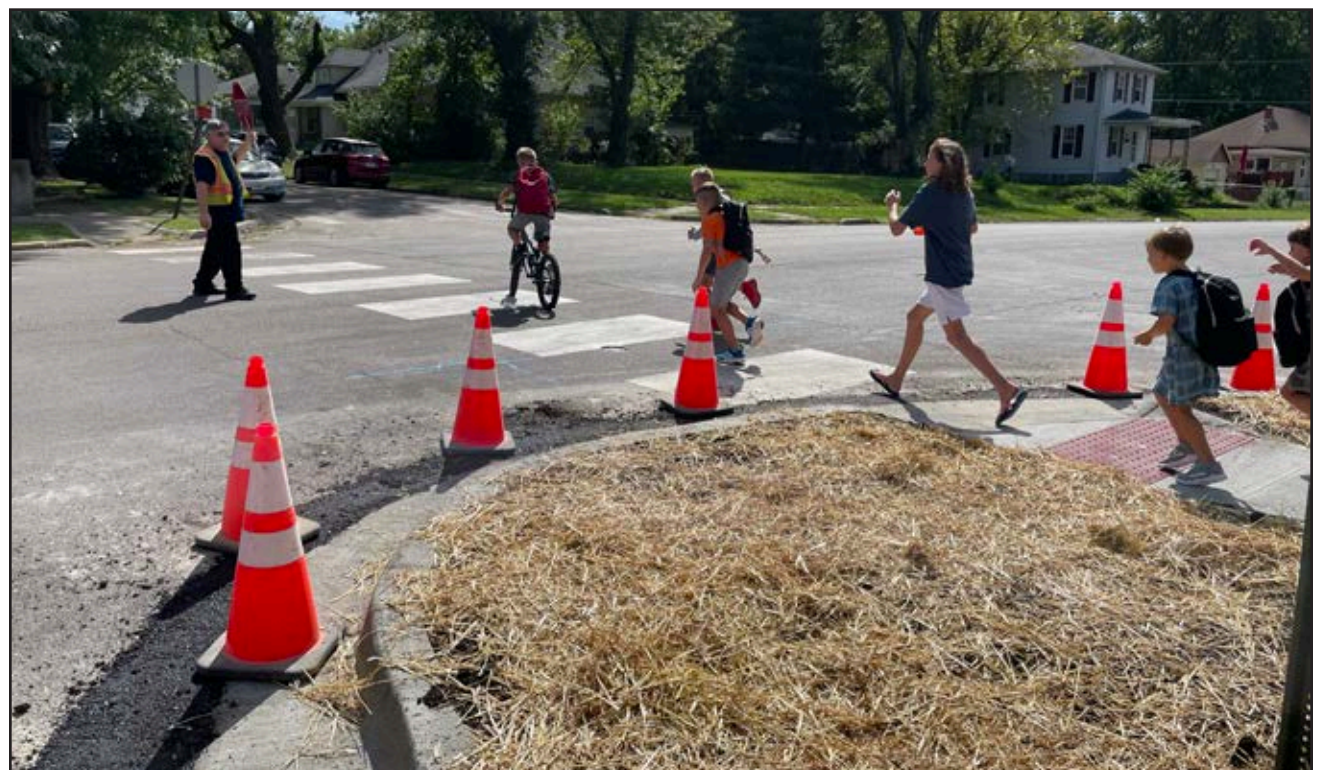
Crossing guard Ernest Lancaster helps pedestrians cross the now-shorter crosswalk on Thursday at Horace Mann Elementary, 1100 W. 16th St. The Sedalia elementary school has new cement bump-outs, islands, and crosswalks to improve pedestrian safety in the new school year.
