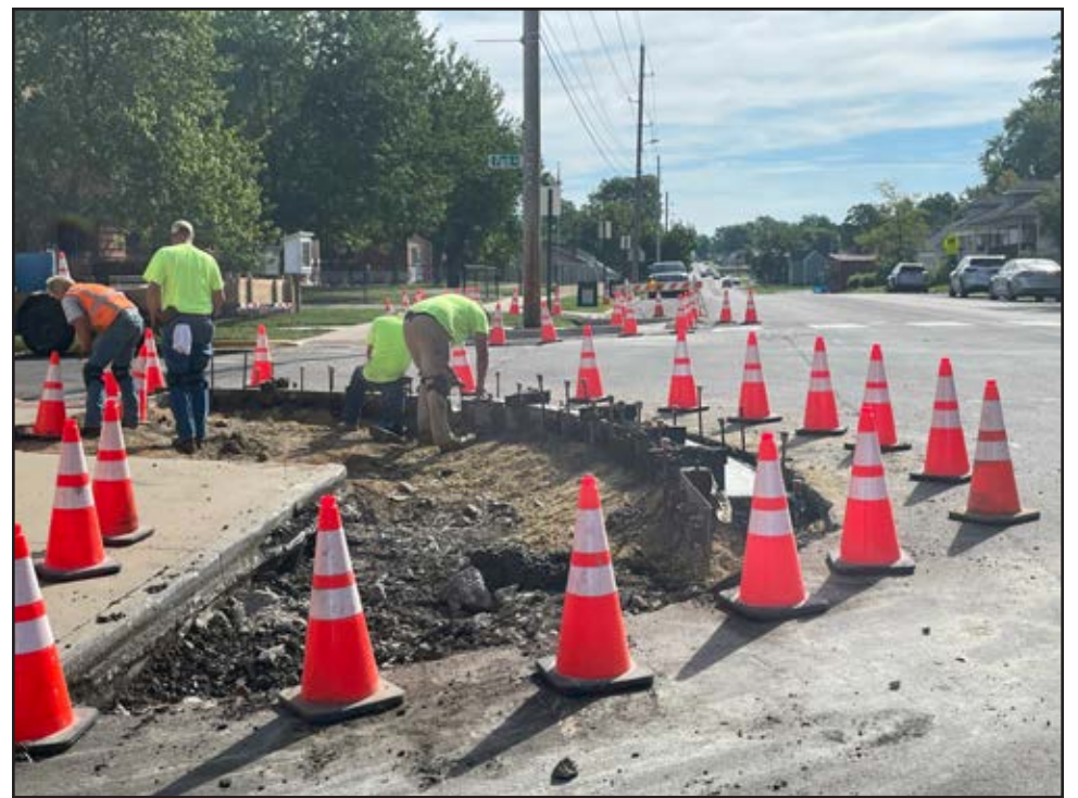
Public Works employees remove cement forms from a bump-out poured Thursday morning. Work has been going on for weeks in front of Horace Mann Elementary and should wrap up soon.
