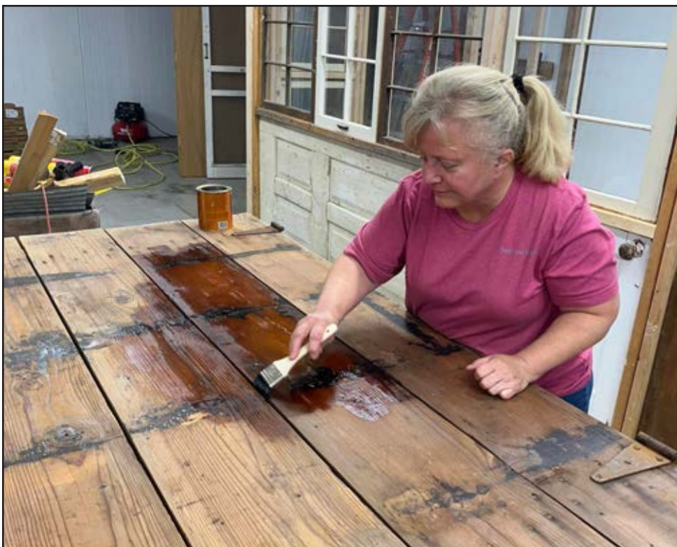
Lisa Dean works on renovations at Bar-B Mercantile's new location at 427 NE Highway 13 in Warrensburg.
