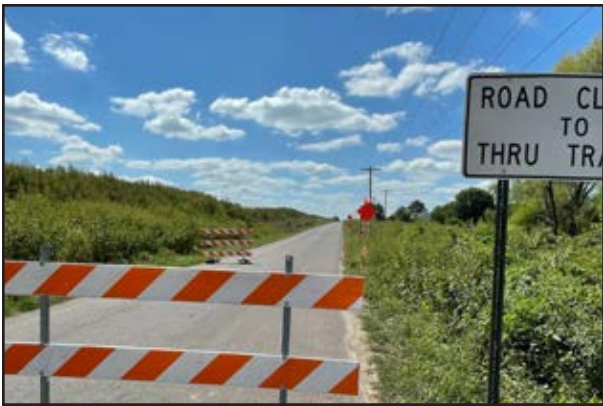
Cedar Drive is closed as crews widen the road. Increased truck traffic is expected along the corridor, especially if Nucor puts in a second entrance on the street.
