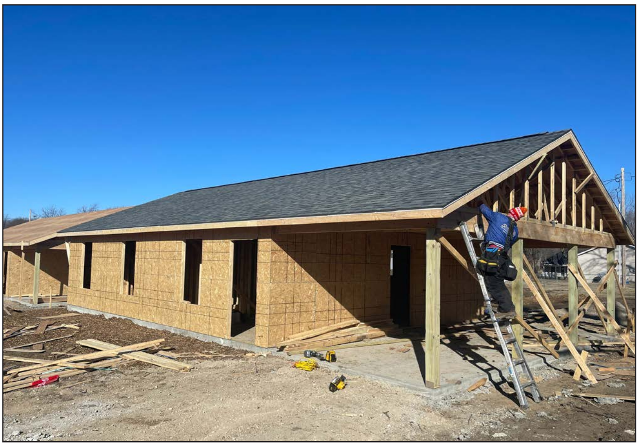
These two Habitat for Humanity homes are being built thanks to a bequest by First Baptist Church member Ethel Hall, whose generous gift now funds two homes per year. Saturday, volunteers are encouraged to bring gloves, tools and lunch.
