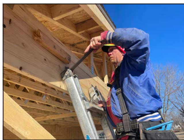
Tony Shepherd with Shep's Construction is teaching carpentry to volunteers working on the Habitat for Humanity home being worked on Saturday in Sedalia.
